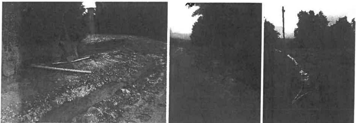
Pictures: The 110 mm sewer diameter damages
