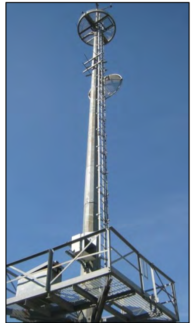
Picture 34: Telkom telephone tower.
