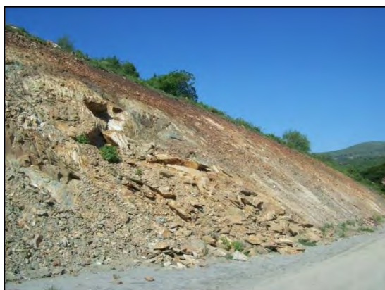
Picture 40: Slope failure in road cutting close to the project site. Upon closer inspection, the failure appears to have occurred as a result of a large wedge failure along mica covered rock joint surfaces.
