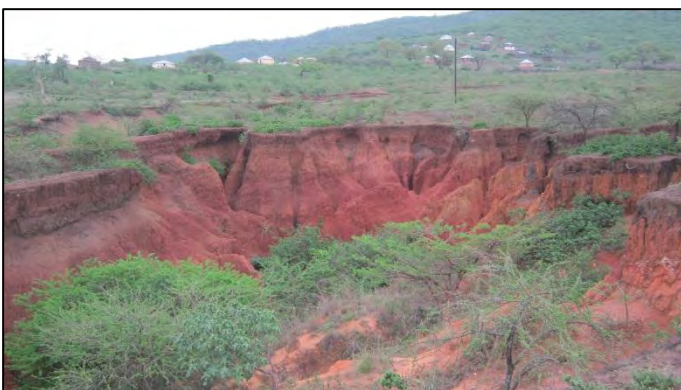
Picture 27: In certain locations, the erosion has become extensive .
