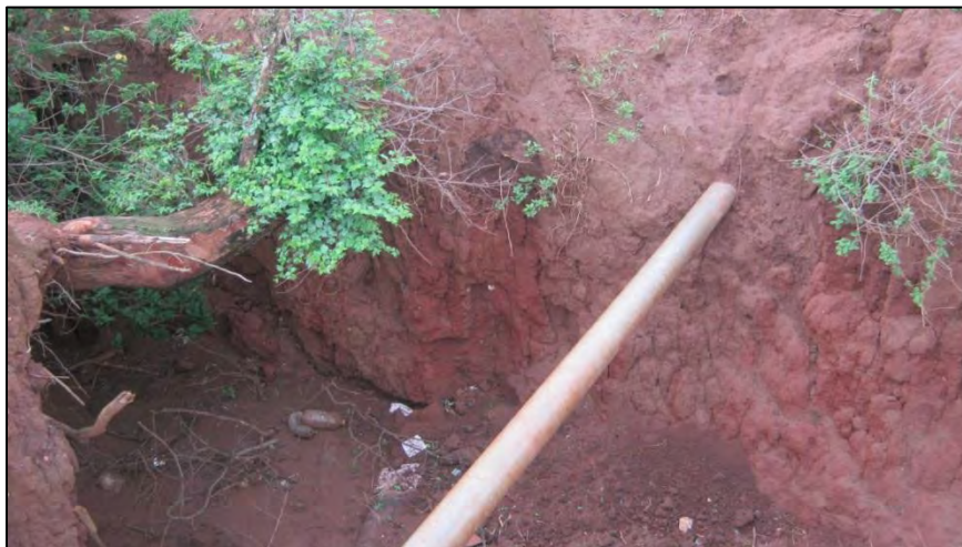
Picture 35: Steel piping used to bridge some of the erosion gullies. The piping of the existing network appears to have become exposed in a number of locations.
