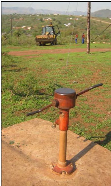
Picture 32: Manually operated borehole pump.
