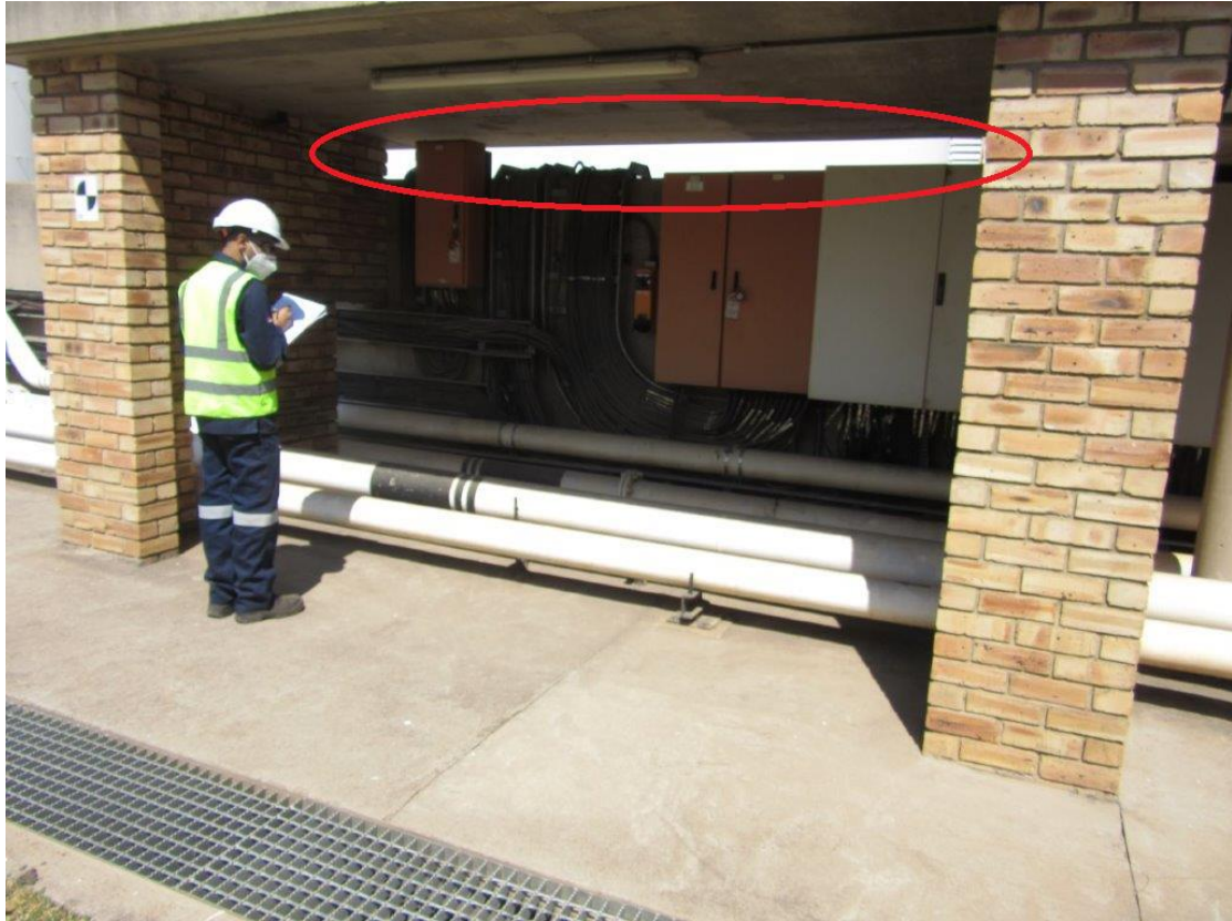
Figure 5: Bund wall local control panel - marked gap to be closed
