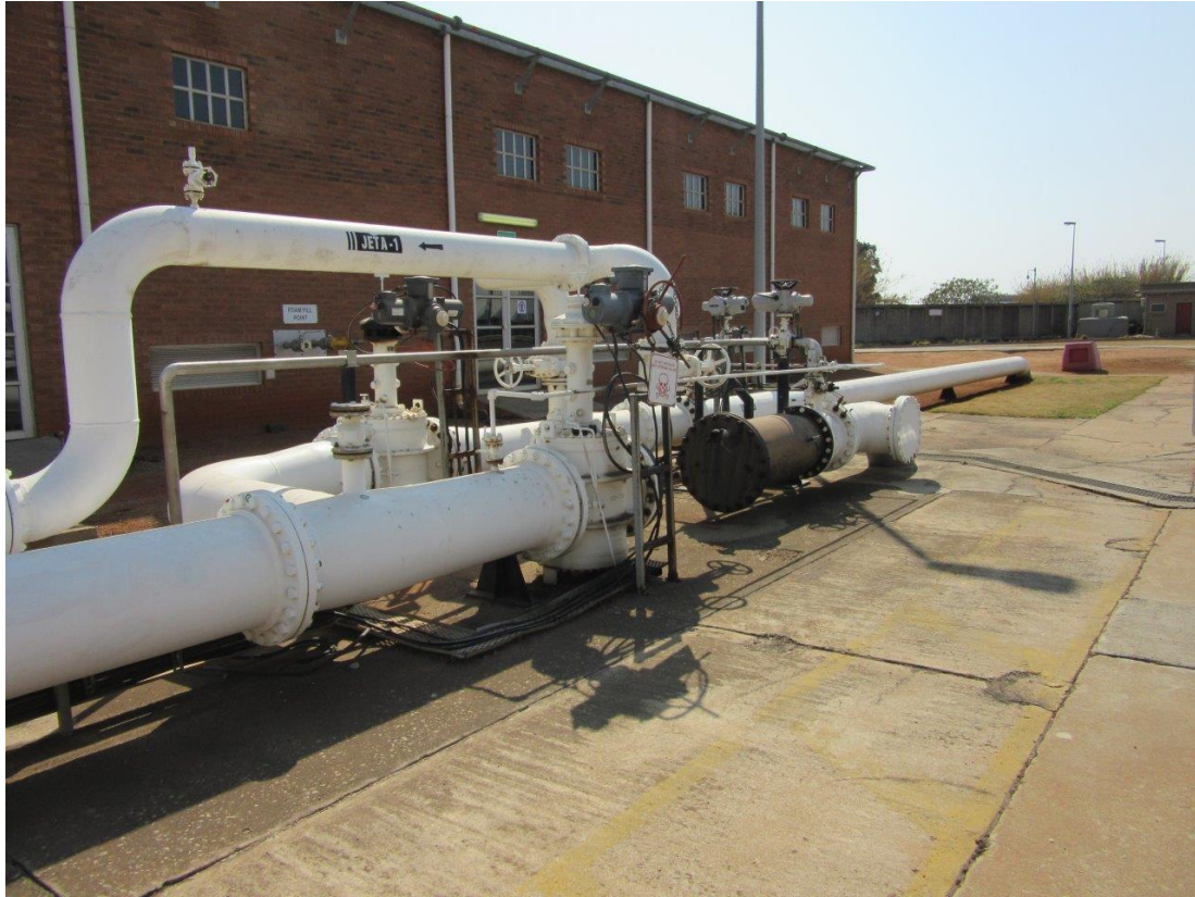
Figure 3: D1 and D2 actuated valves (D2 de-commissioned)
