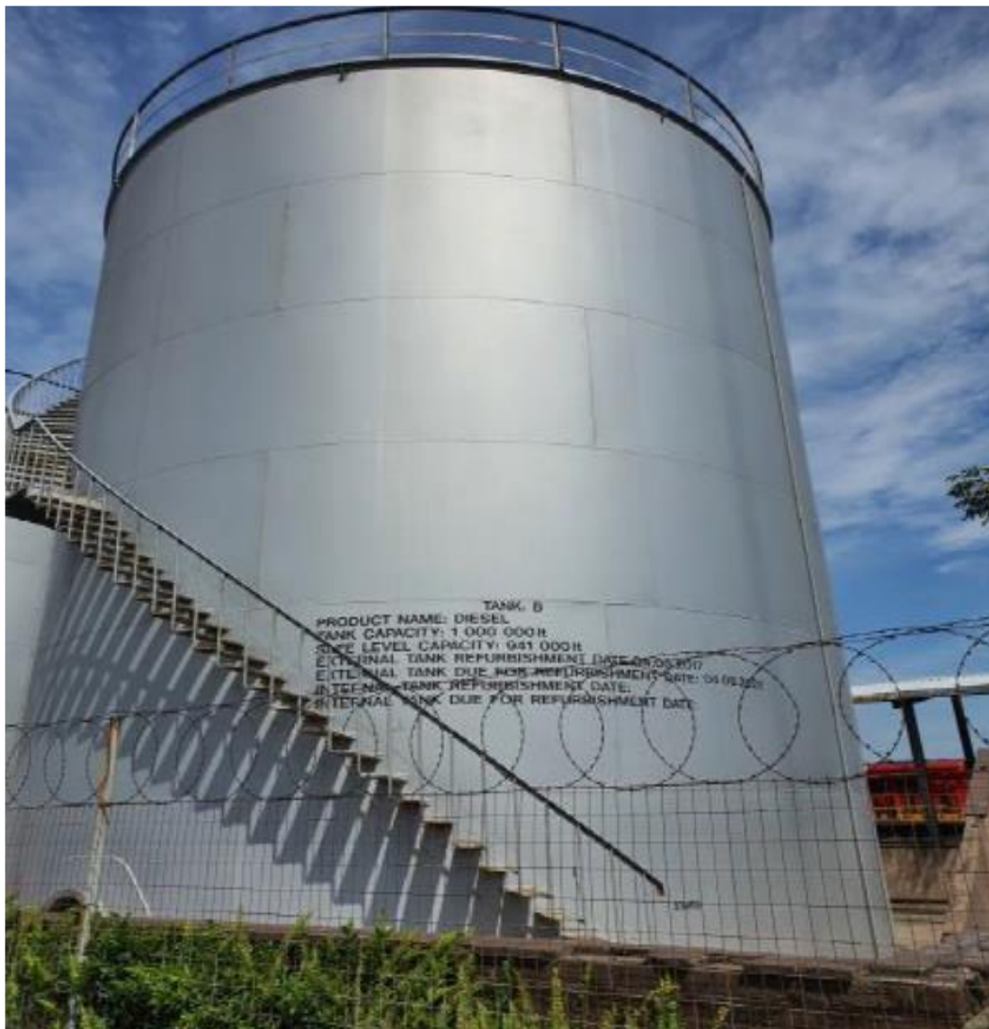
Wentworth Tank-(Height 11.94m, Diameter 10.02m and Capacity 941m 3 )
