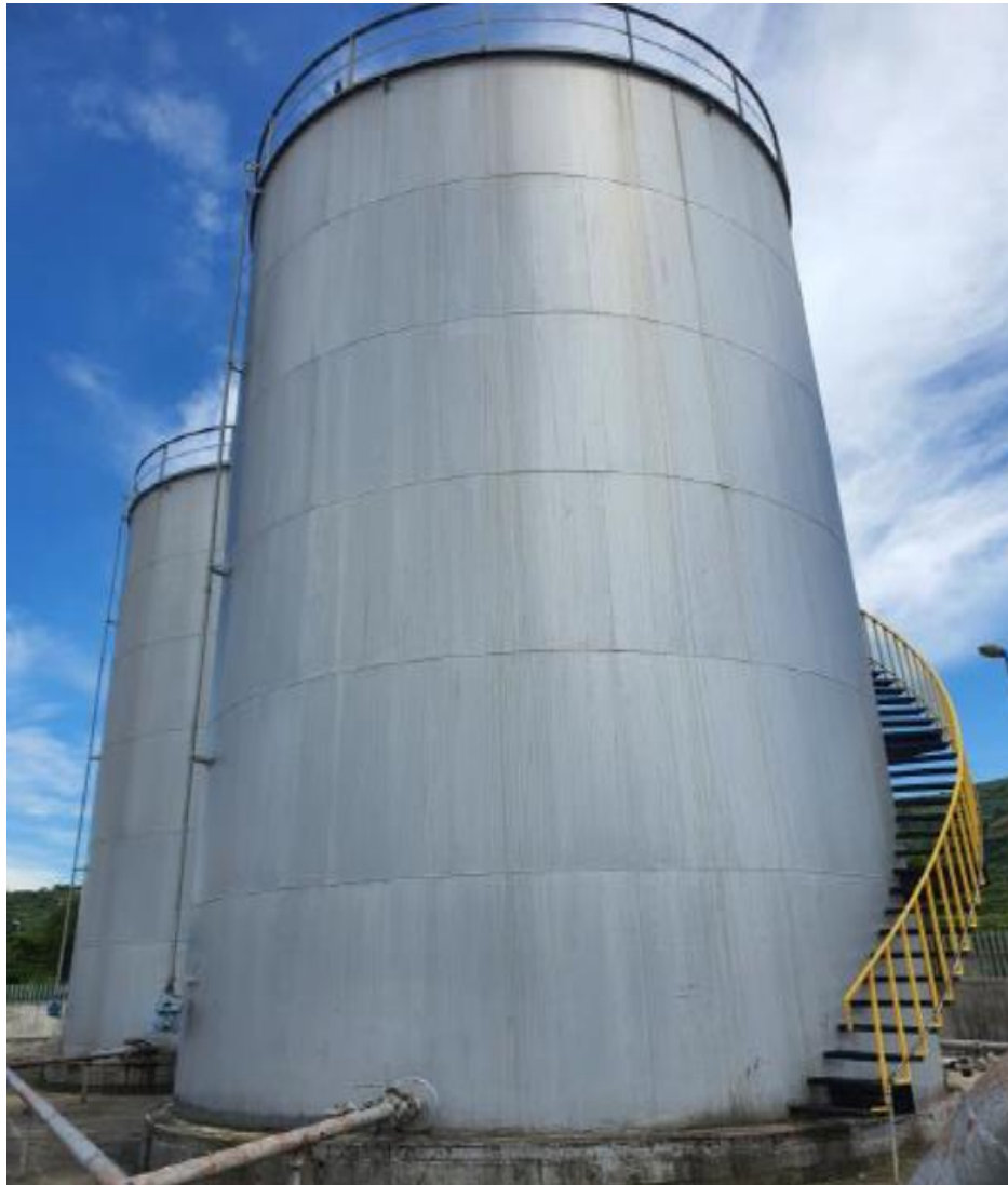
Masons Mill Tank (Height 11.93m, Diameter 7.52m and Capacity 529.6m 3 )
