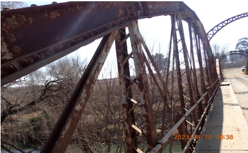
View on rusting on steel sections
