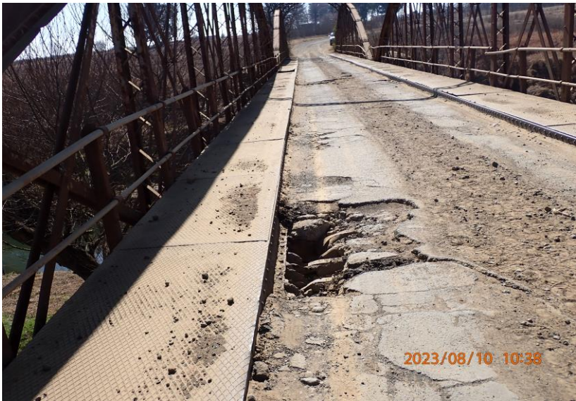
View on damaged deck
