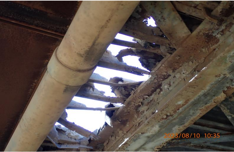
View on damaged deck
