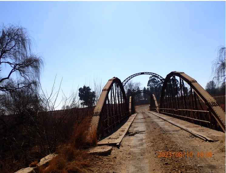
View on bridge and missing sections on truss
