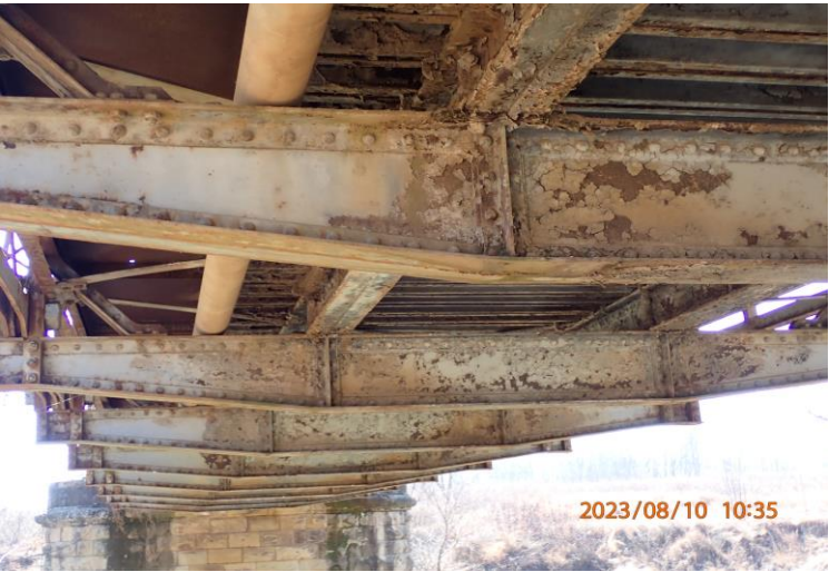
View on corroded deck sections
