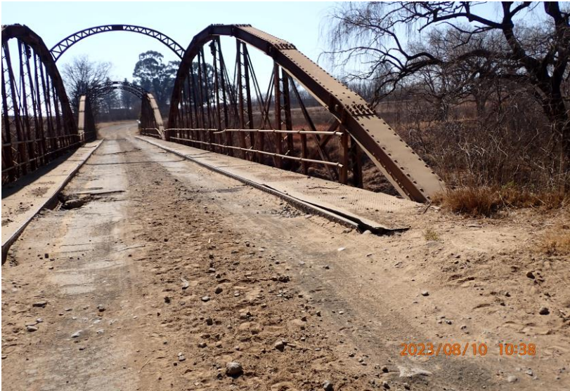
Rusting on deck sections and damaged walkway
