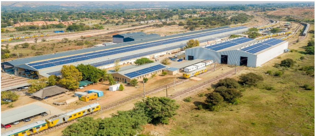
Existing 1 (ONE) MW Solar roof top plant
