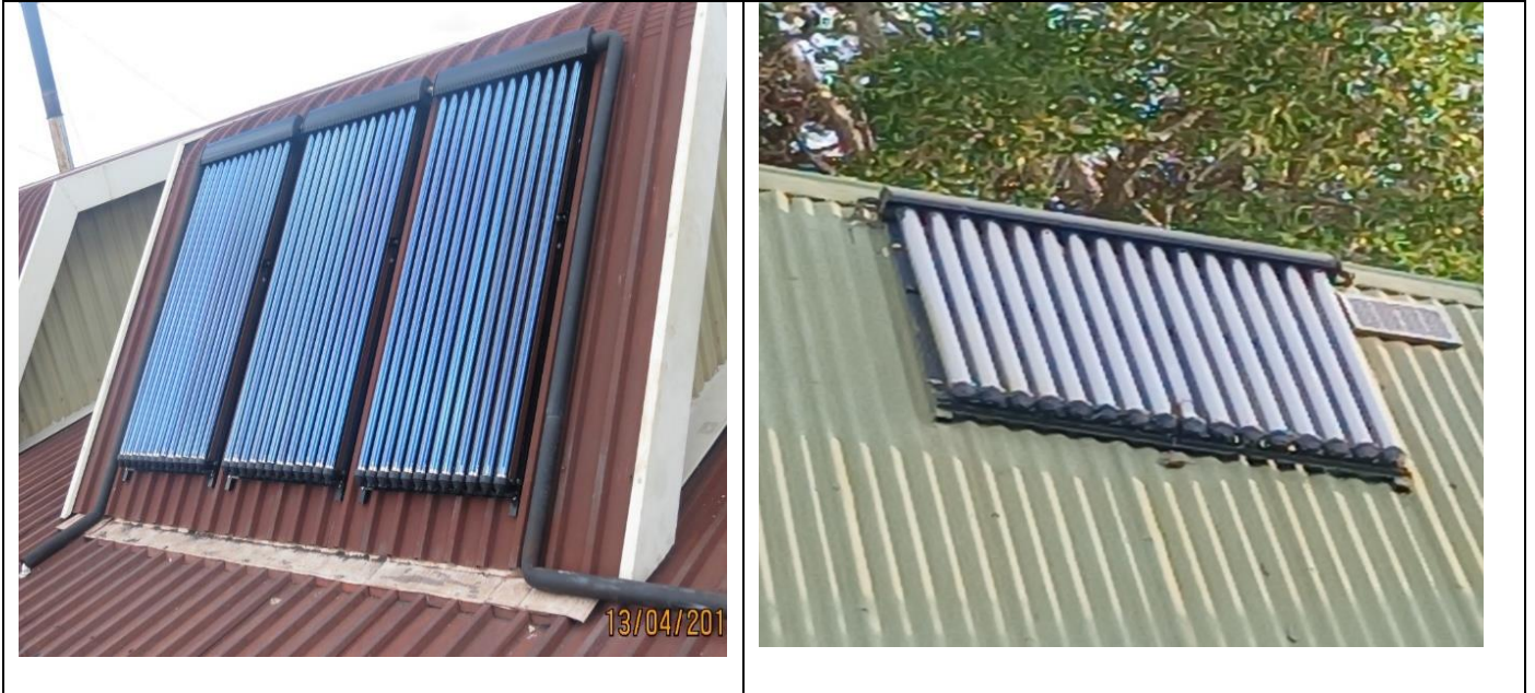
Photo 4: Existing Old Solar Geyser Installation System (Note most Geysers are inside the building, and Circulation Pump)
