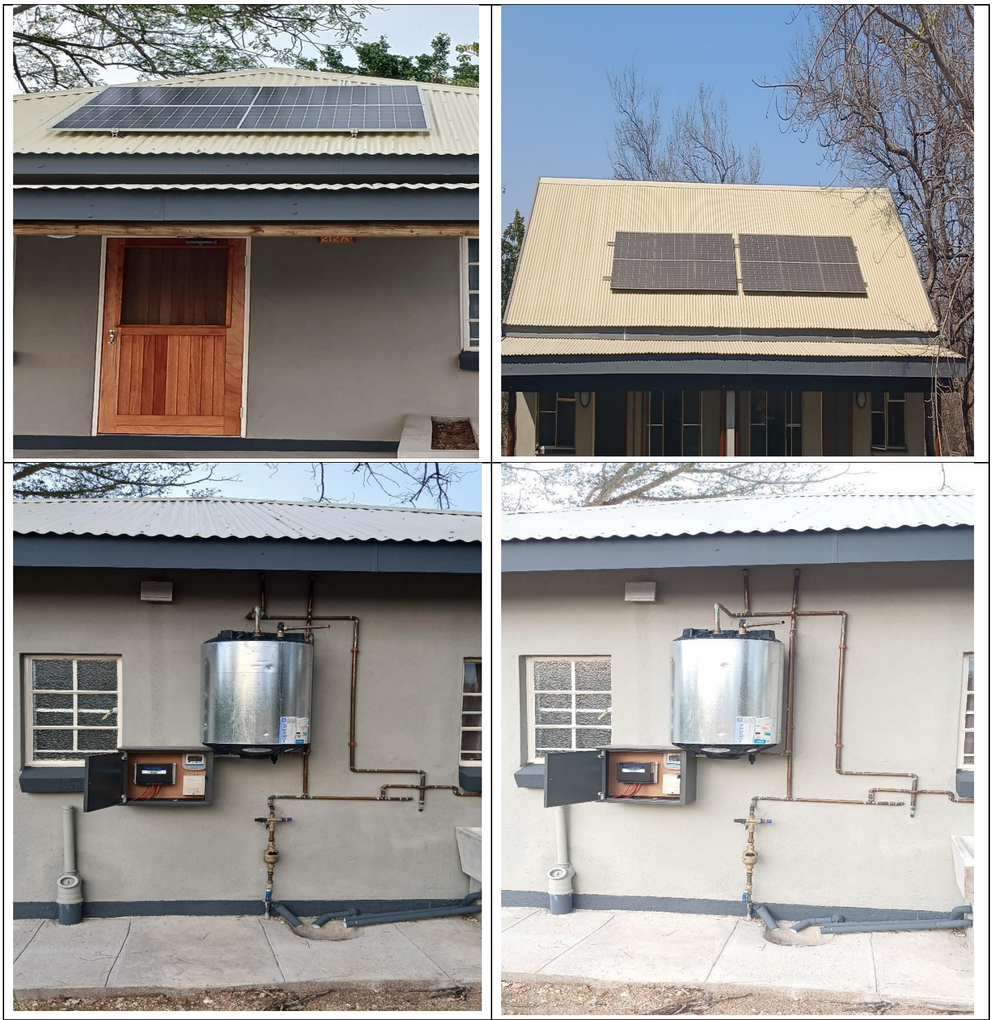
Photo 2: New Existing Solar Geyser (Geysers are moved Outside and Solar panels can be anywhere suitable close by)
