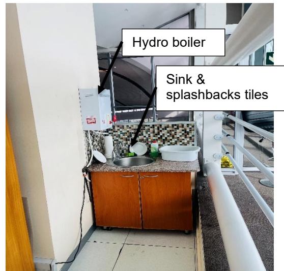
Figure 2: Current sink and hydro boiler location
