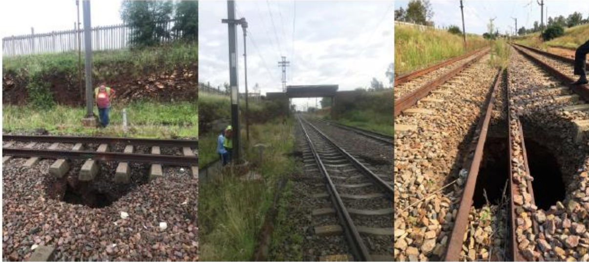
Figure 1: The re-occurrence of sinkholes in the Pinedene station area, WA Km 35 to 36
