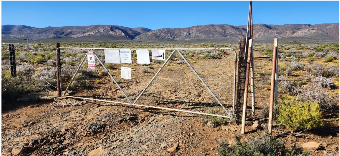
Figure 3: Existing outer perimeter gate to be replaced.
