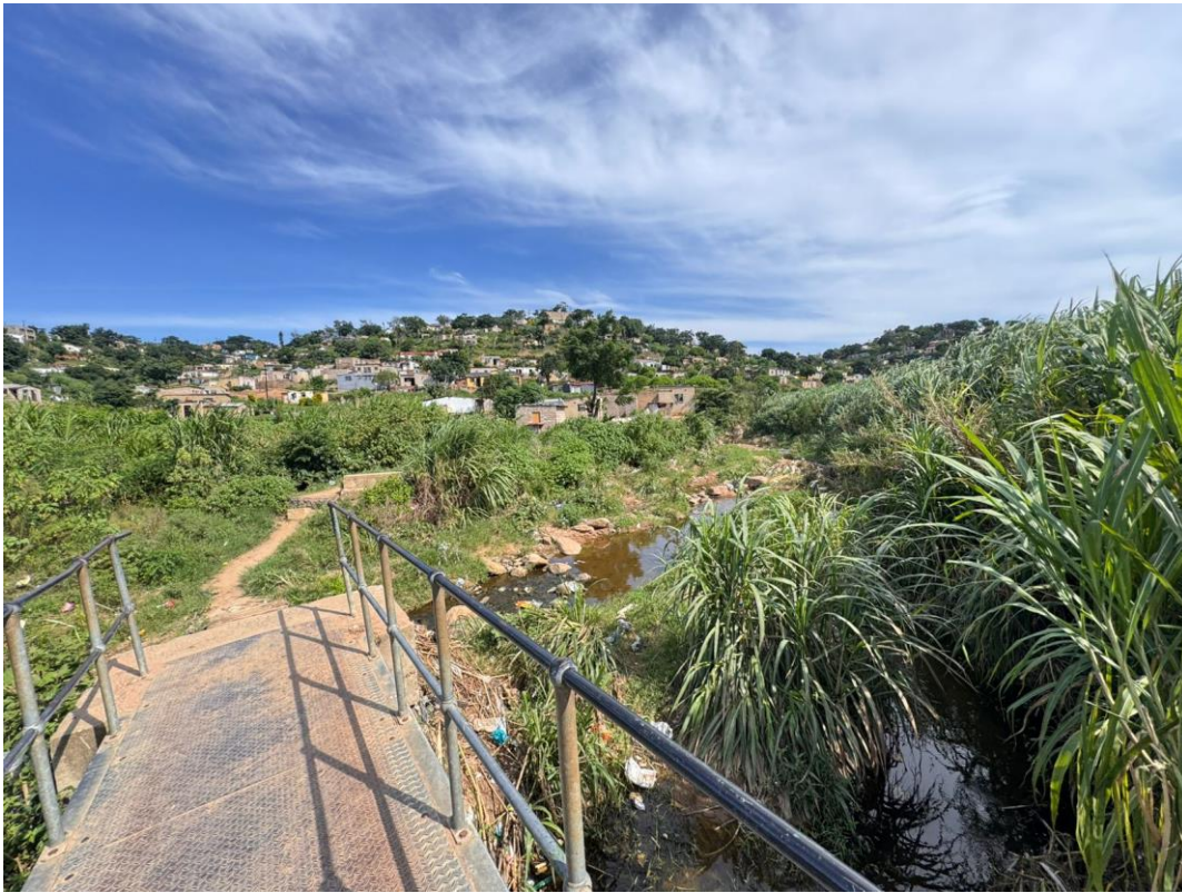
Figure 2: An existing 12m steel pedestrian bridge, accommodating half of the river stream length, and illegal dumping next to the bridge.
