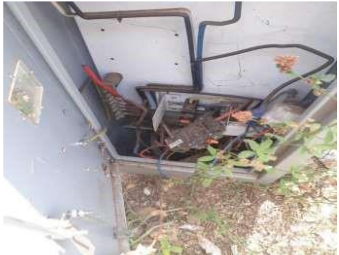
Picture 2: Vandalised electrical works at the station
