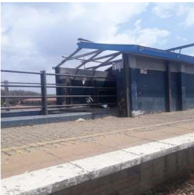
Picture 3: Vandalised structure at the station
