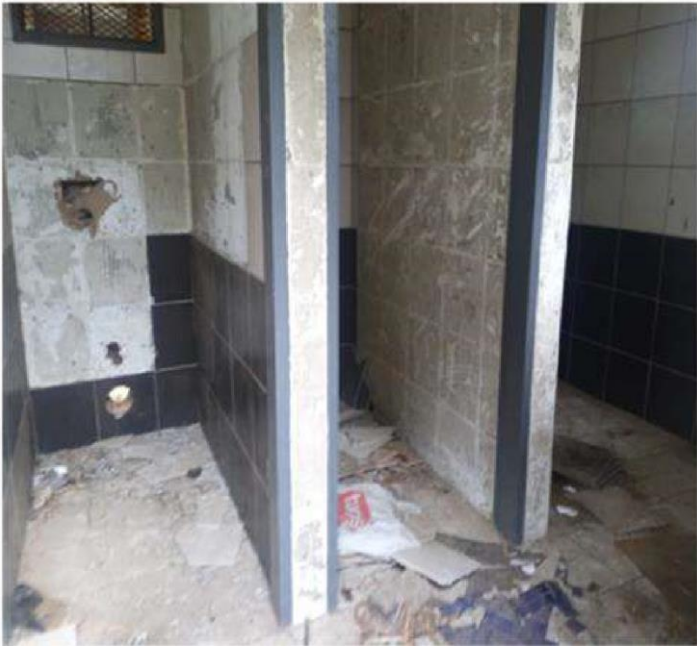
Picture 1: Vandalised ablutions at the station
