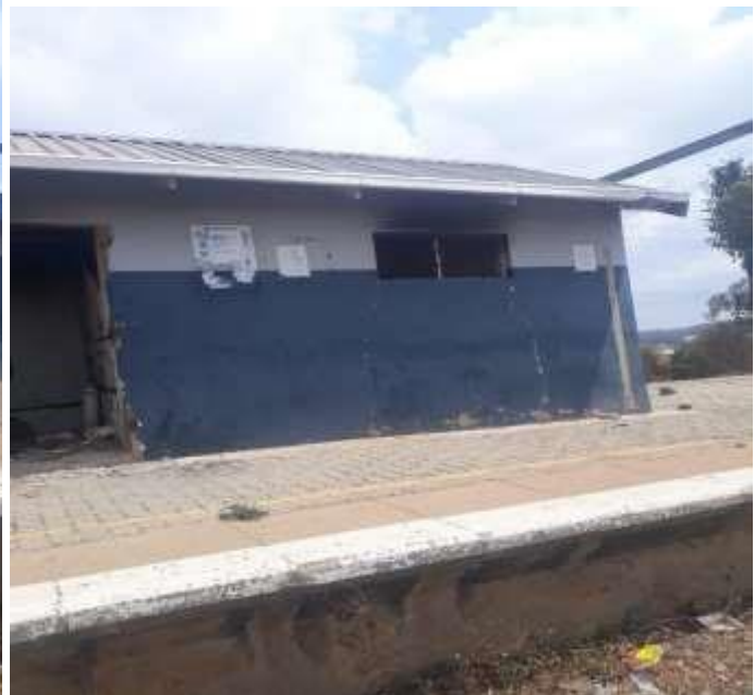
Picture 4: Vandalised structure at the station
