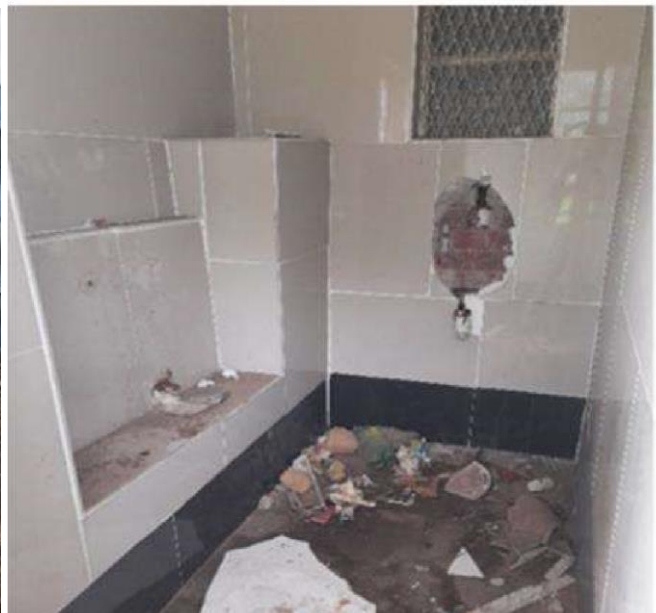
Picture 4: Vandalised toilets at the station
