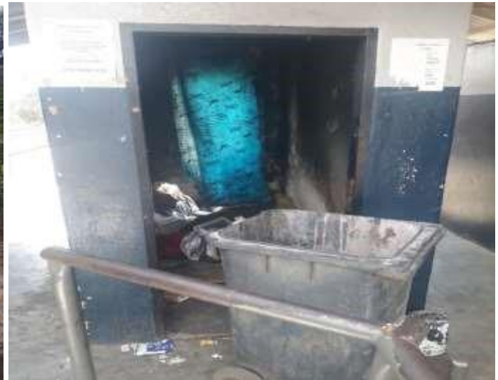
Picture 2: Dilapidated structure at the station
