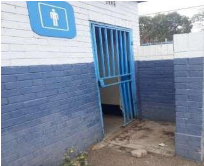
Picture 1: Vandalised toilets at the station
