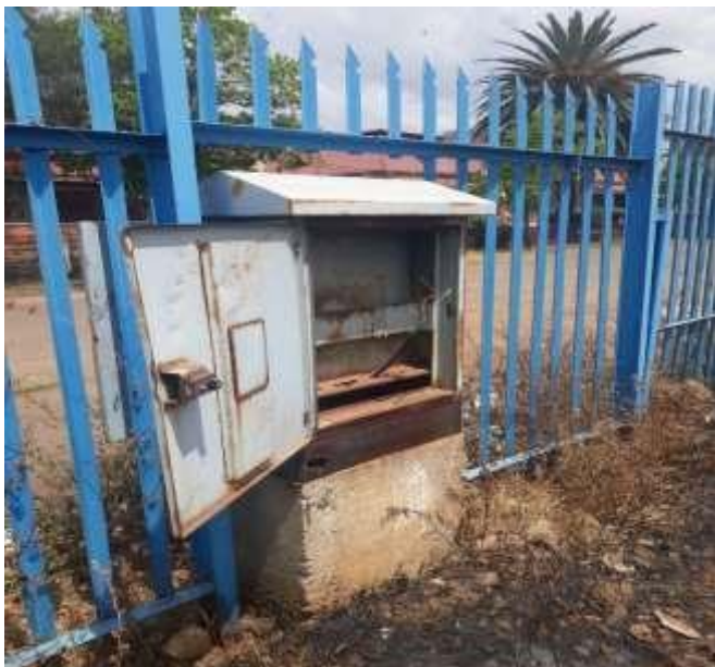
Picture 3: Vandalised electrical works at the station
