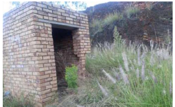
Picture 4: Vandalised structure at the station
