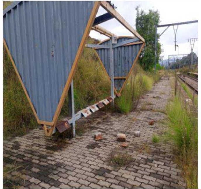
Picture 2: Dilapidated shelters at the station
