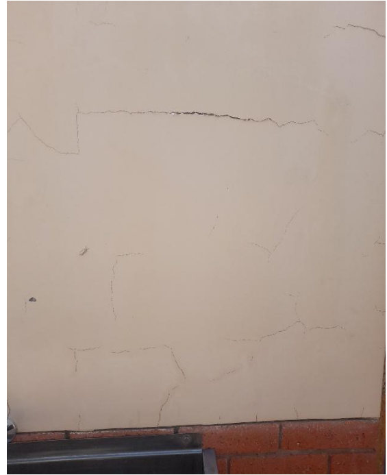
Fig 2: Cracks in plaster
