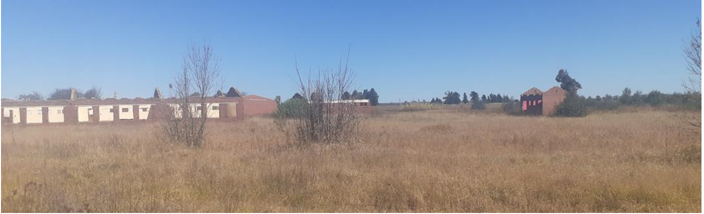
Figure 3: Existing Dilapidated structures on site
