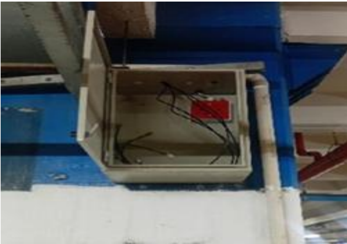
Figure 27: ORTIA MSP1 and 2 (Existing Housing to be used)
