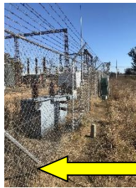
Concrete Slab pre-cast cable cover from Feeder Breaker to the first pole (BD1)
