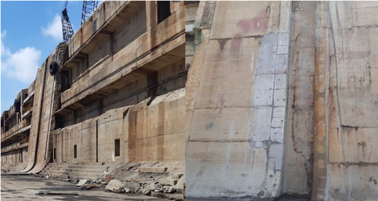
Figure 7: Spalled Concrete and Repairs to Dock Gate Groove
