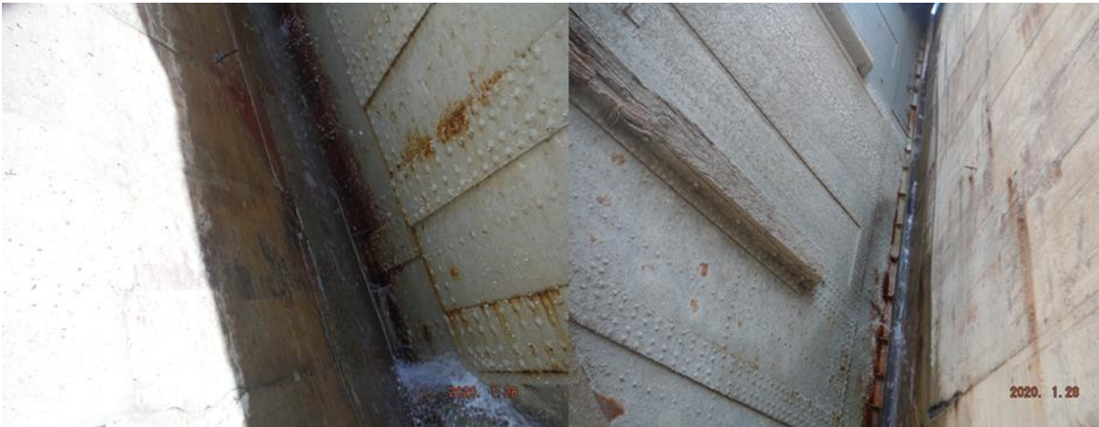
Figure 8: Leaks at Dock Gate Grooves
