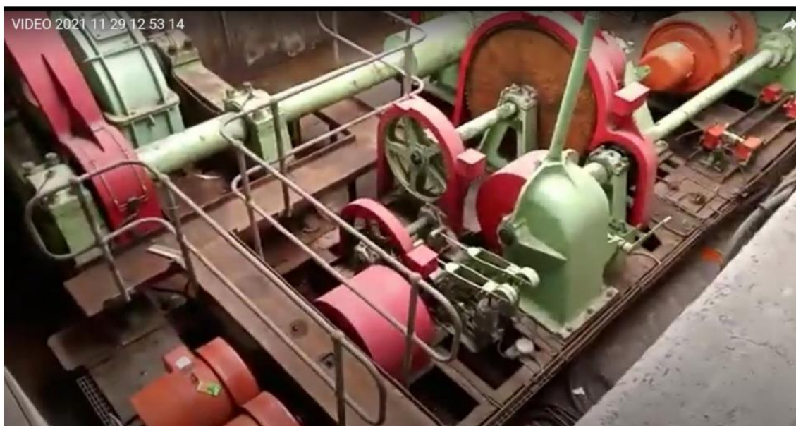
Figure 6 Winch House (Caisson Drive Train)
