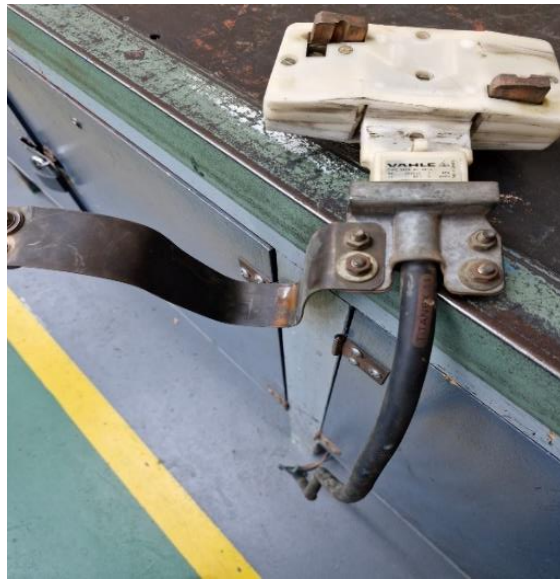
Figure 2: Damaged current carrier front view
