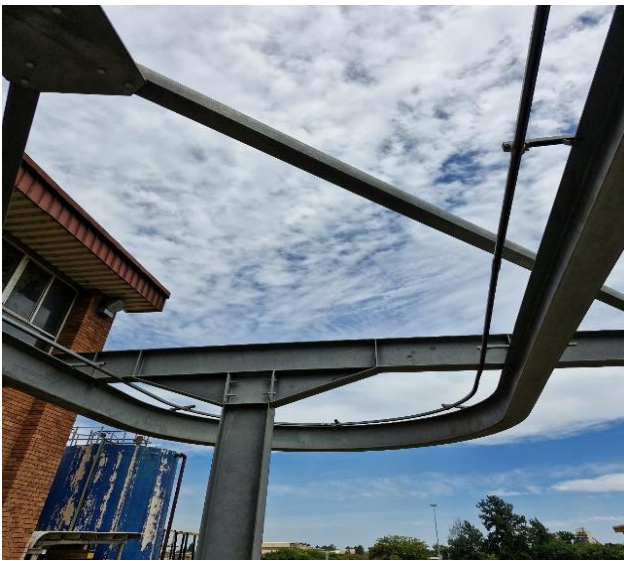
Figure 4: Damaged C- Track curve
