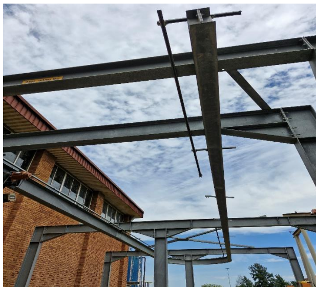
Figure 5: Missing C- Track portions
