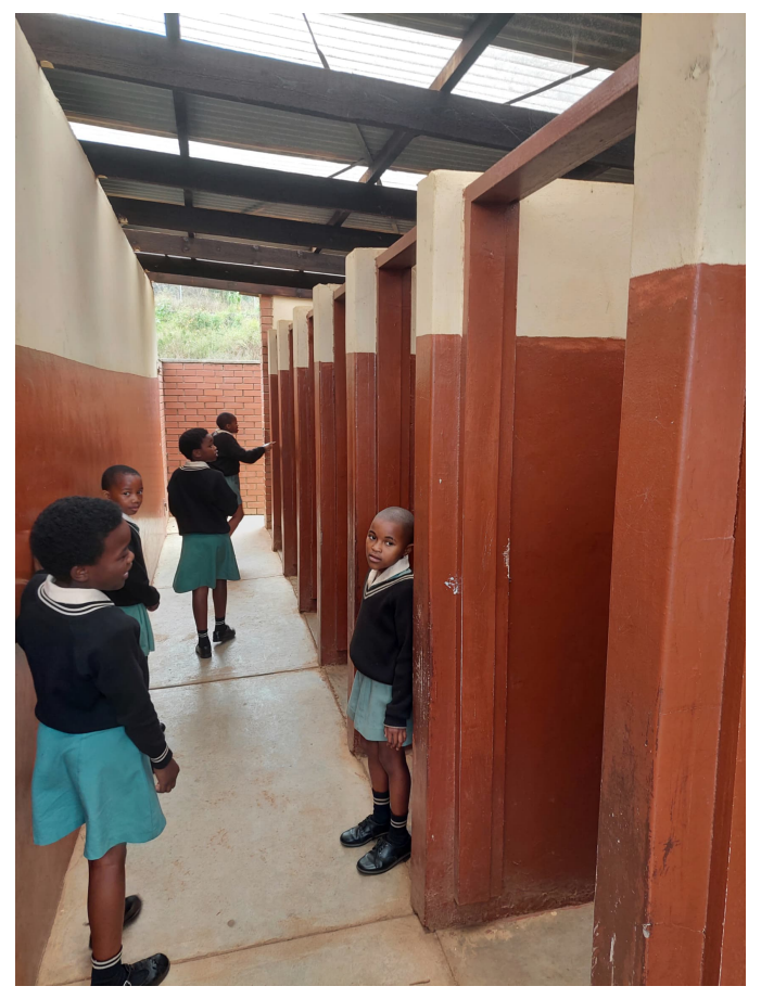
Figure 1 & 2: Interior images of the girls bathroom showing damaged toilet fittings and the roof sheeting. The painted walls show signs of age
