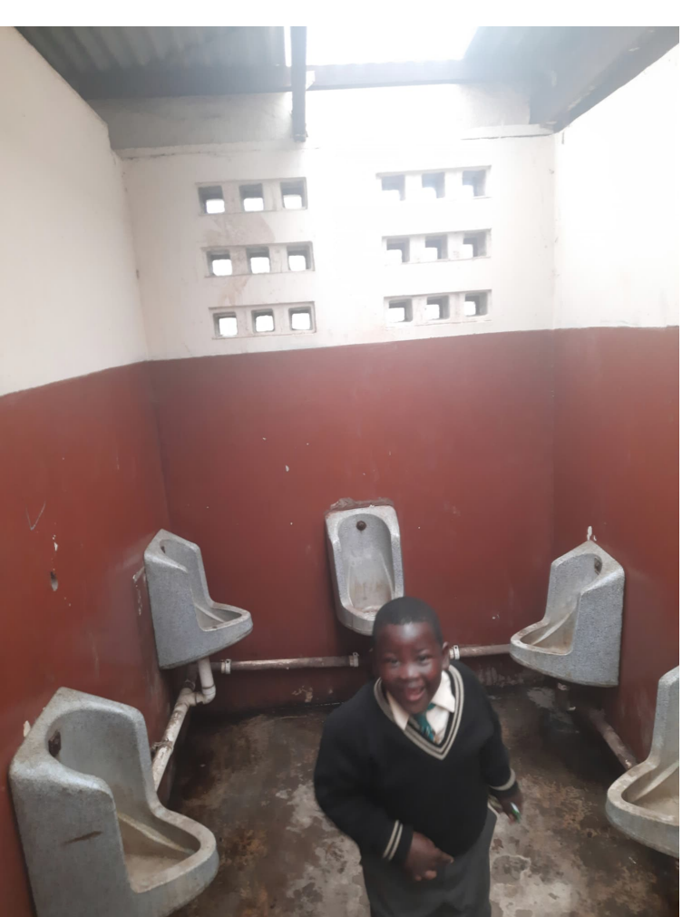
Figure 5: Interior of Boys ablutions. The urinals are in poor condition and would need to be replaced. The concrete floors are also in a bad condition
