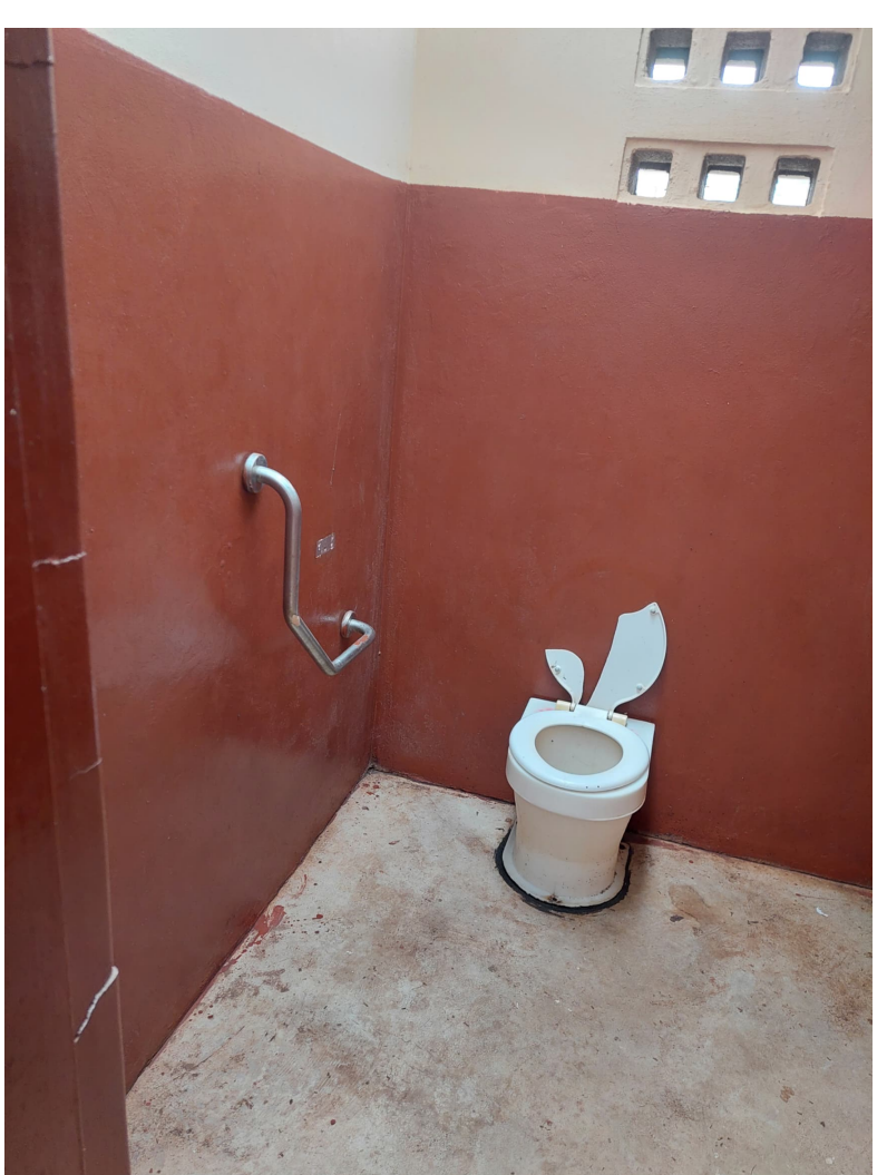
Figure 6: Interior image of the damaged disabled toilet in the female ablutions, this cubicle will be converted into a female toilet
