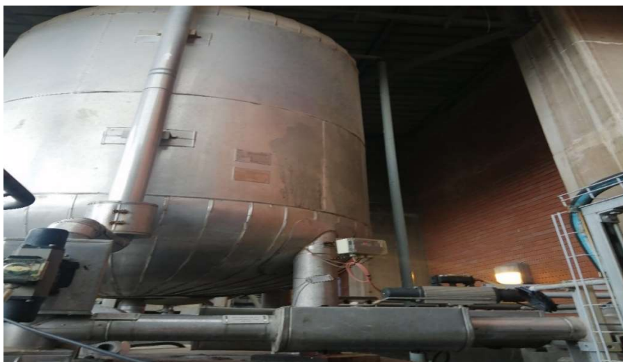
Figure 8: CPP regen caustic measure tank, vent line connected back to the caustic bulk storage tank.
