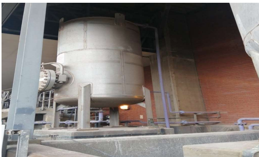
Figure 7: Sulfuric acid measure tank vent line to the sulfuric acid bulk storage tank.
