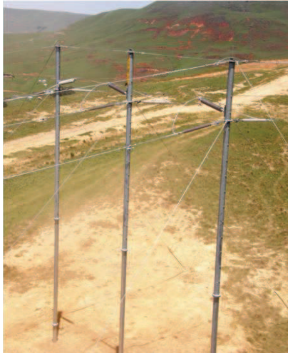
Figure-5 : Steel Trips monopole strain structure (D-DT-7618)
