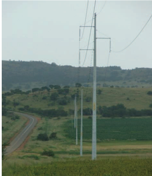
Figure 3: Self supporting monopole suspension structures (D-DT-7649)
