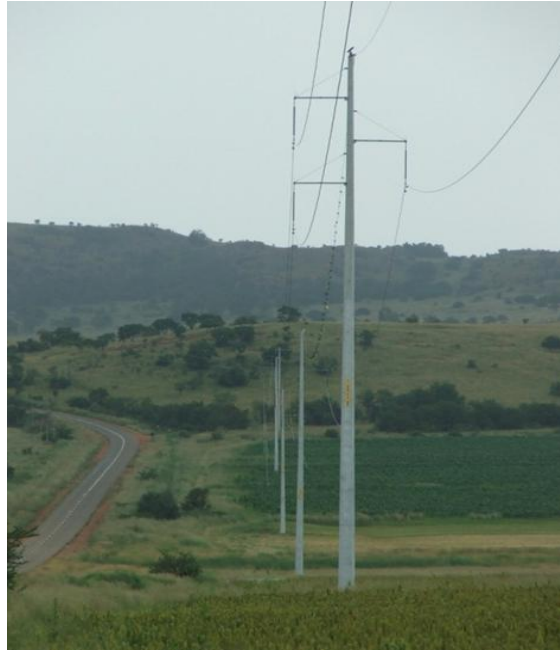
Figure 3: Self supporting monopole suspension structures (D-DT-7649)
