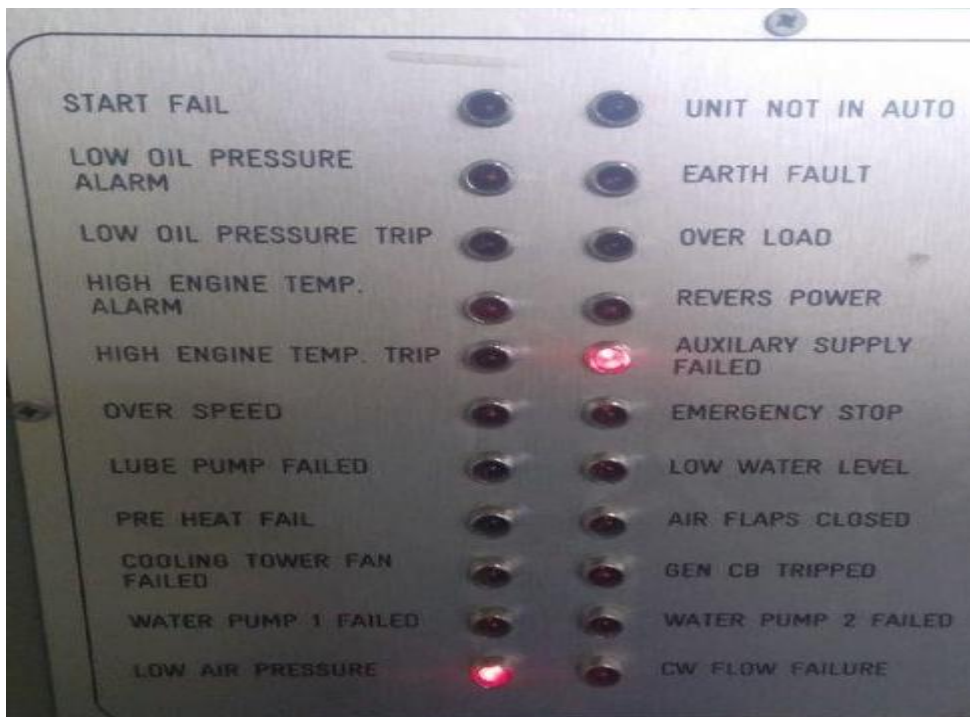
Figure 3: Current signals on 380V Diesel Generator Control Panels
