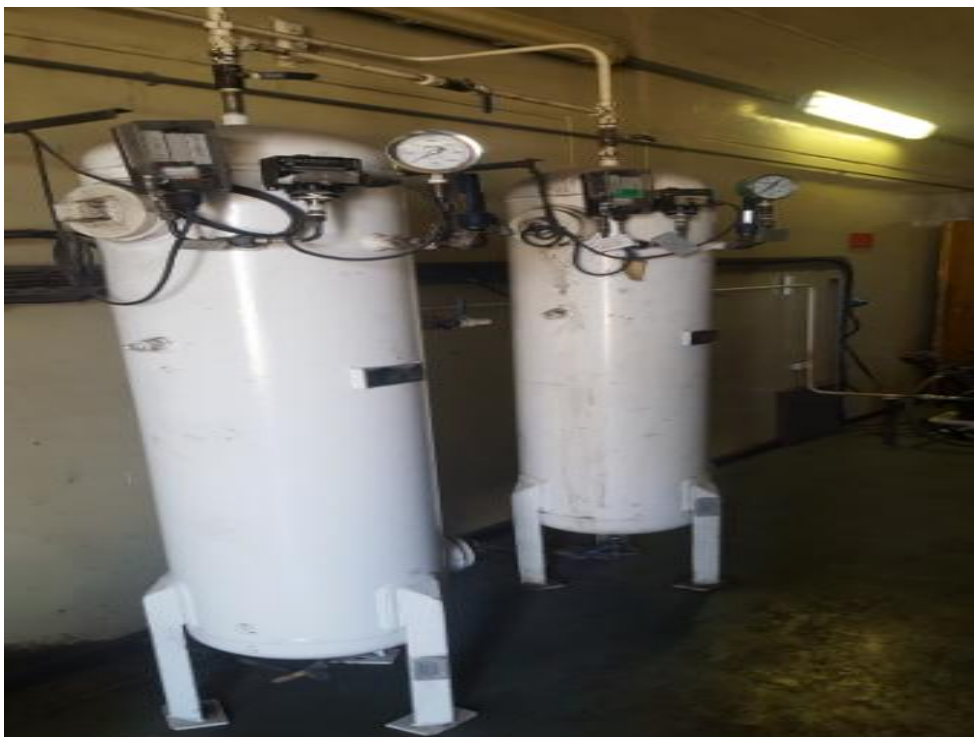
Figure 5: Existing Air Receivers
