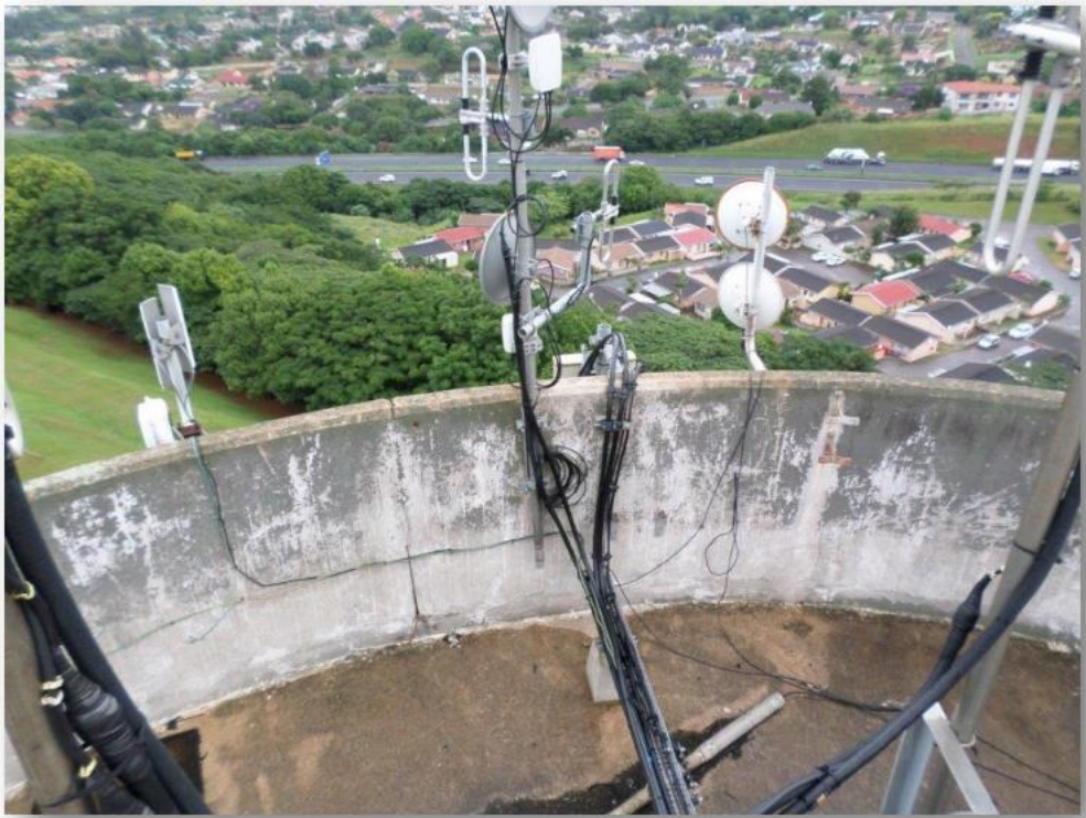
6M Pole on top of the Water tower
