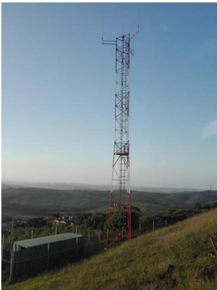
36M Lattice Tower
