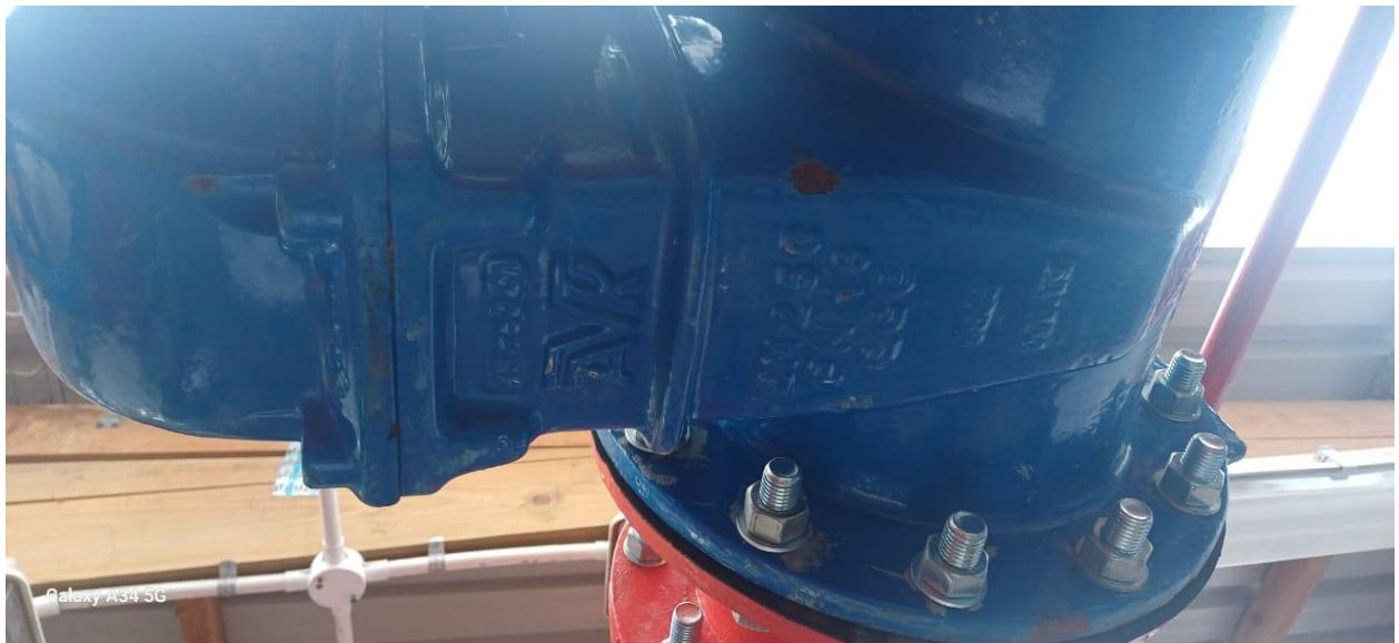
Main Discharge Valve
