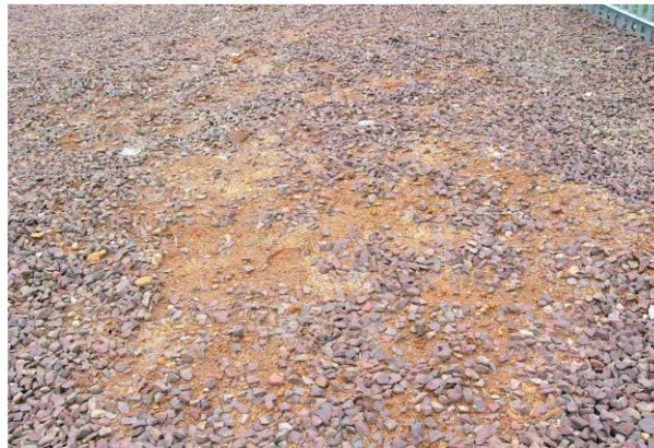
Figure 14: Exposed soil due to poor workmanship
