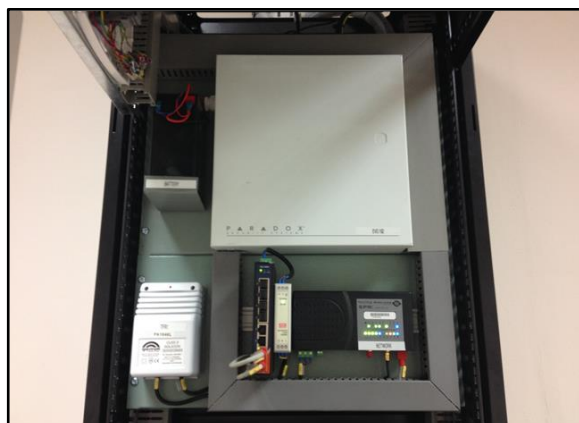
Figure 8: Example of Well Organised Security Equipment Cabinet
