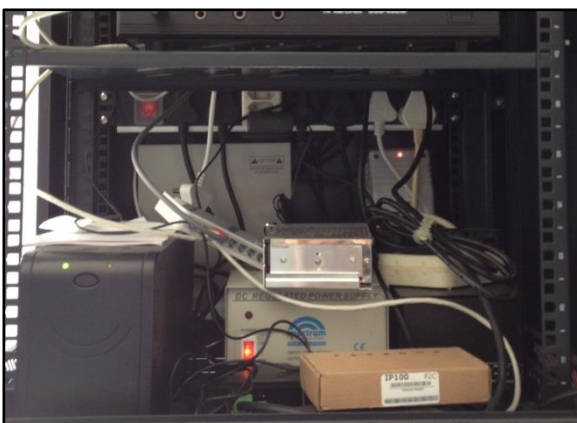
Figure 7: Example of Poorly Organised Security Equipment Cabinet
