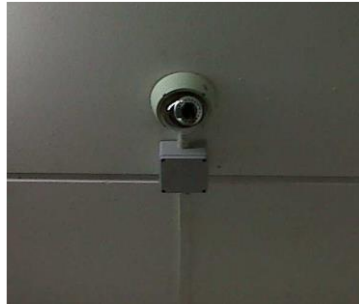
Figure 17: Indoor camera inside room
