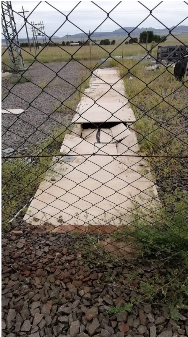
Image 1: Trench covers at Rouxville sub
