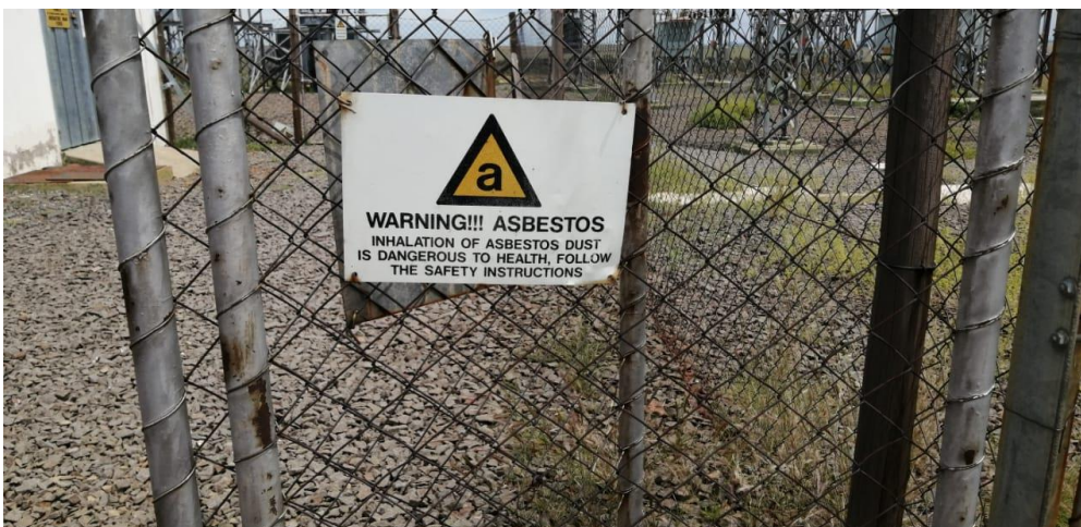
Image 2: Asbestos warning signs on fence at Rouxville sub
