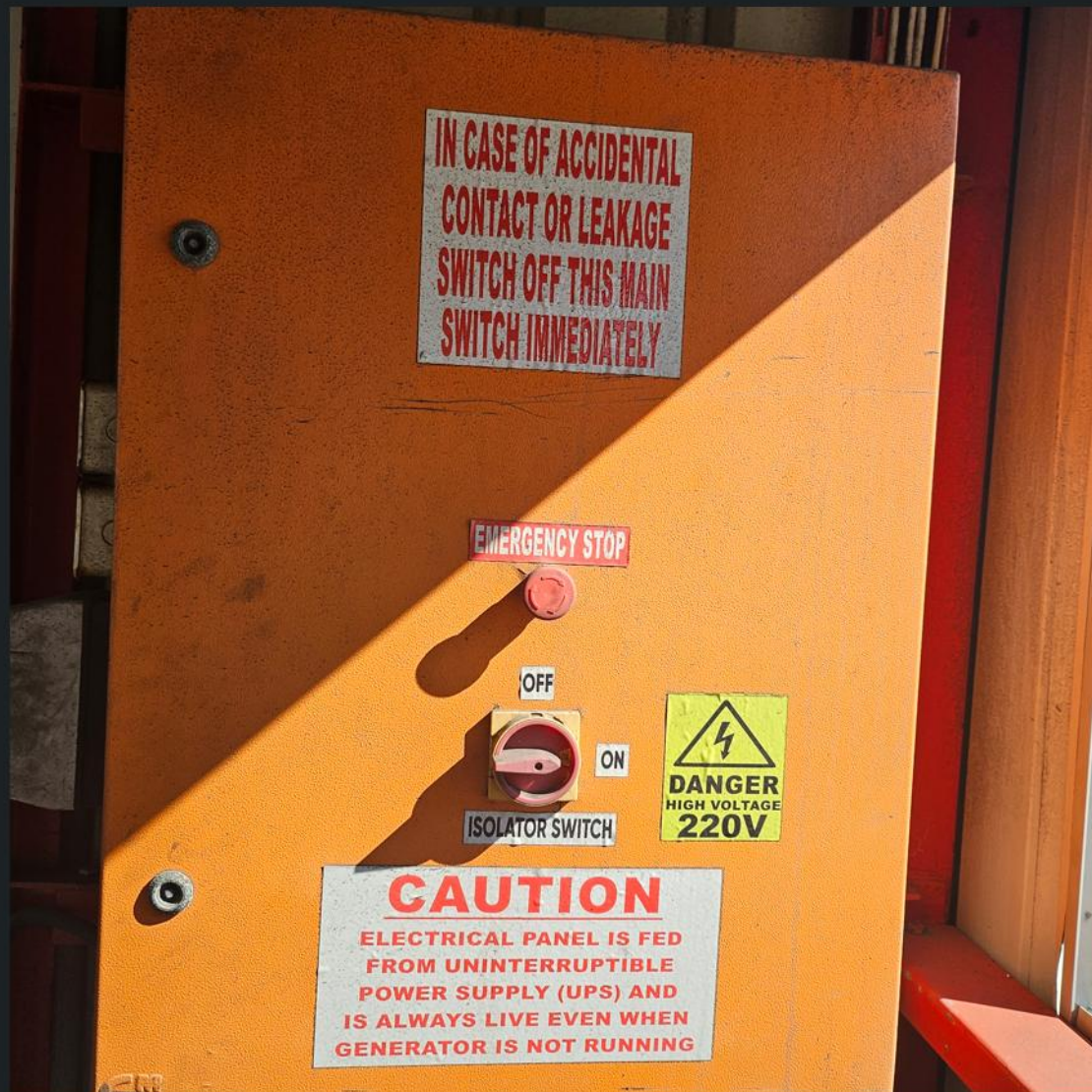
Pump Electrical Box.jpg
