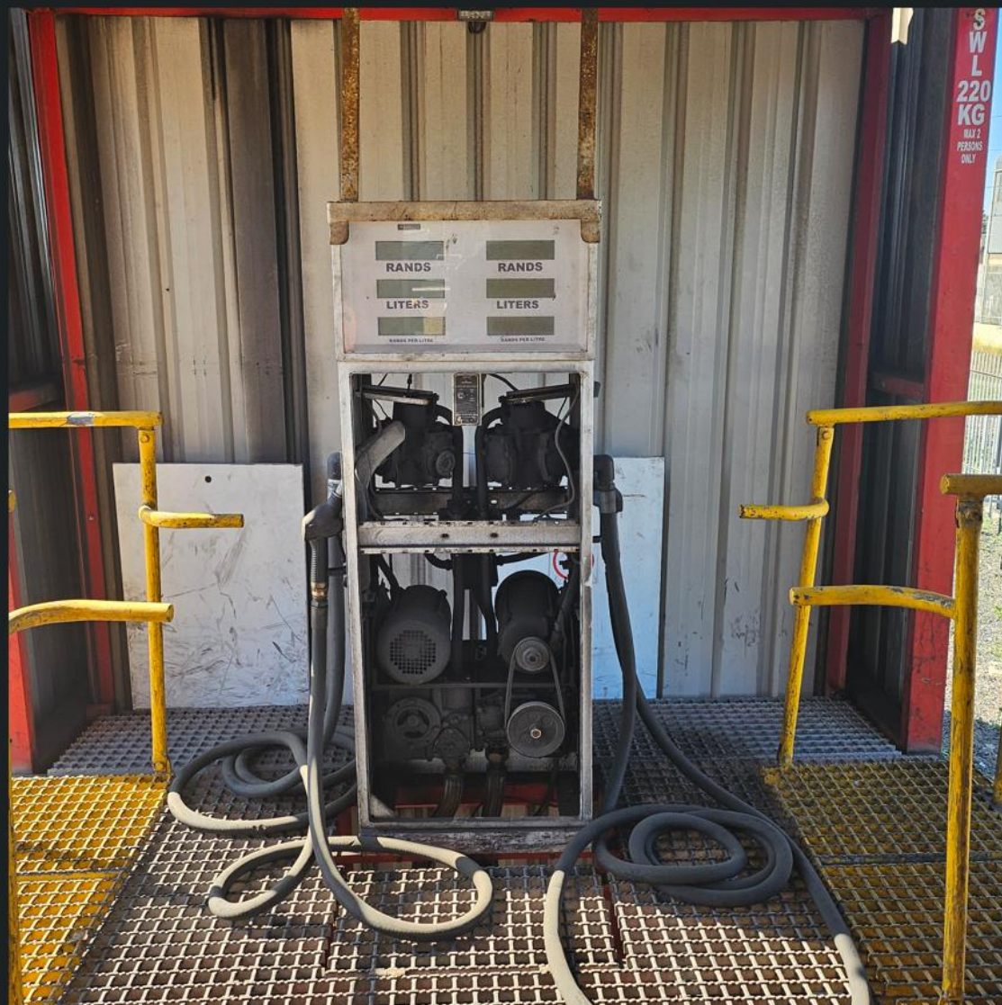
Dispenser Pump - Pic 2.jpg
