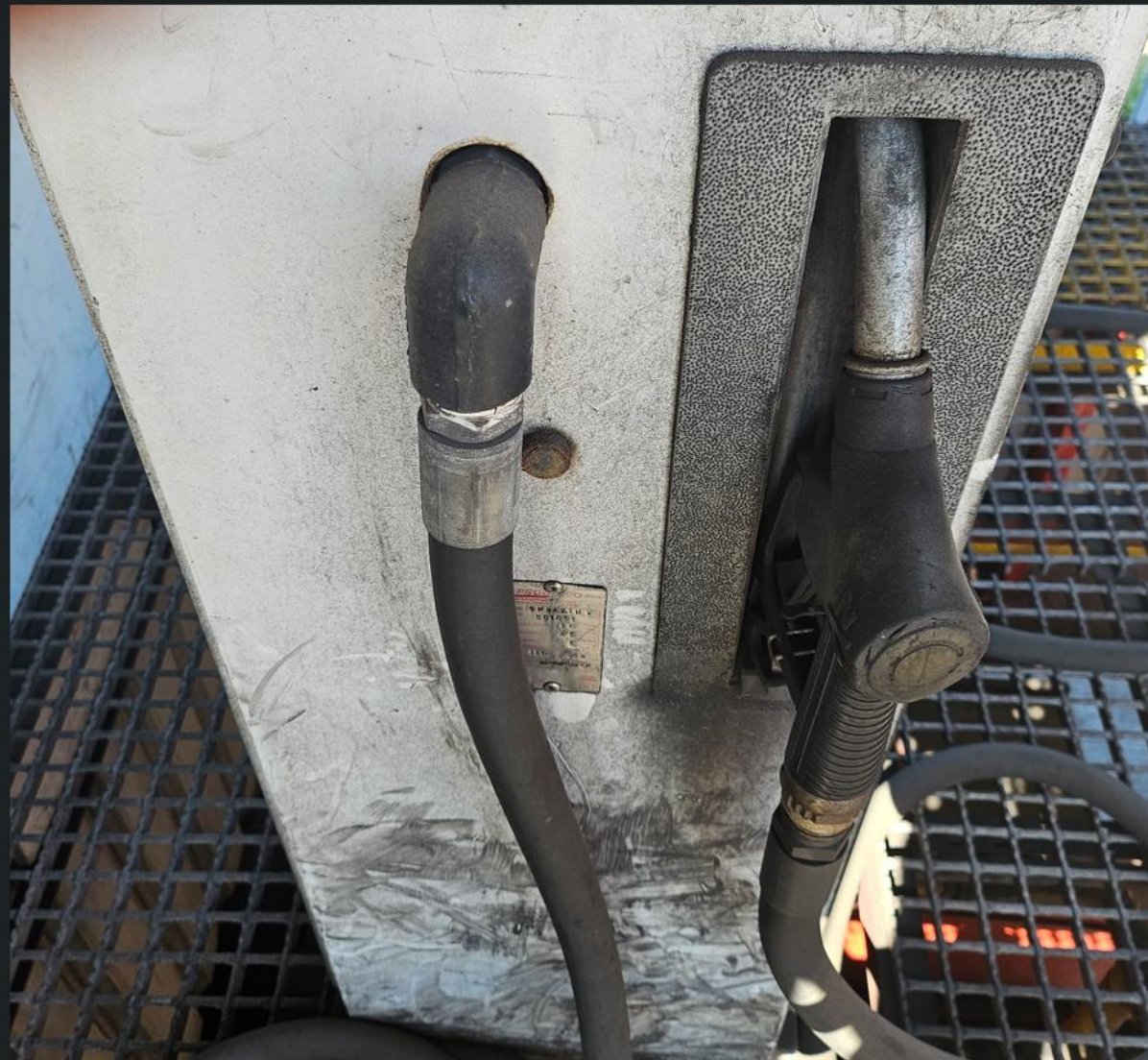
Dispenser Pump - LHS Nozzle.jpg
