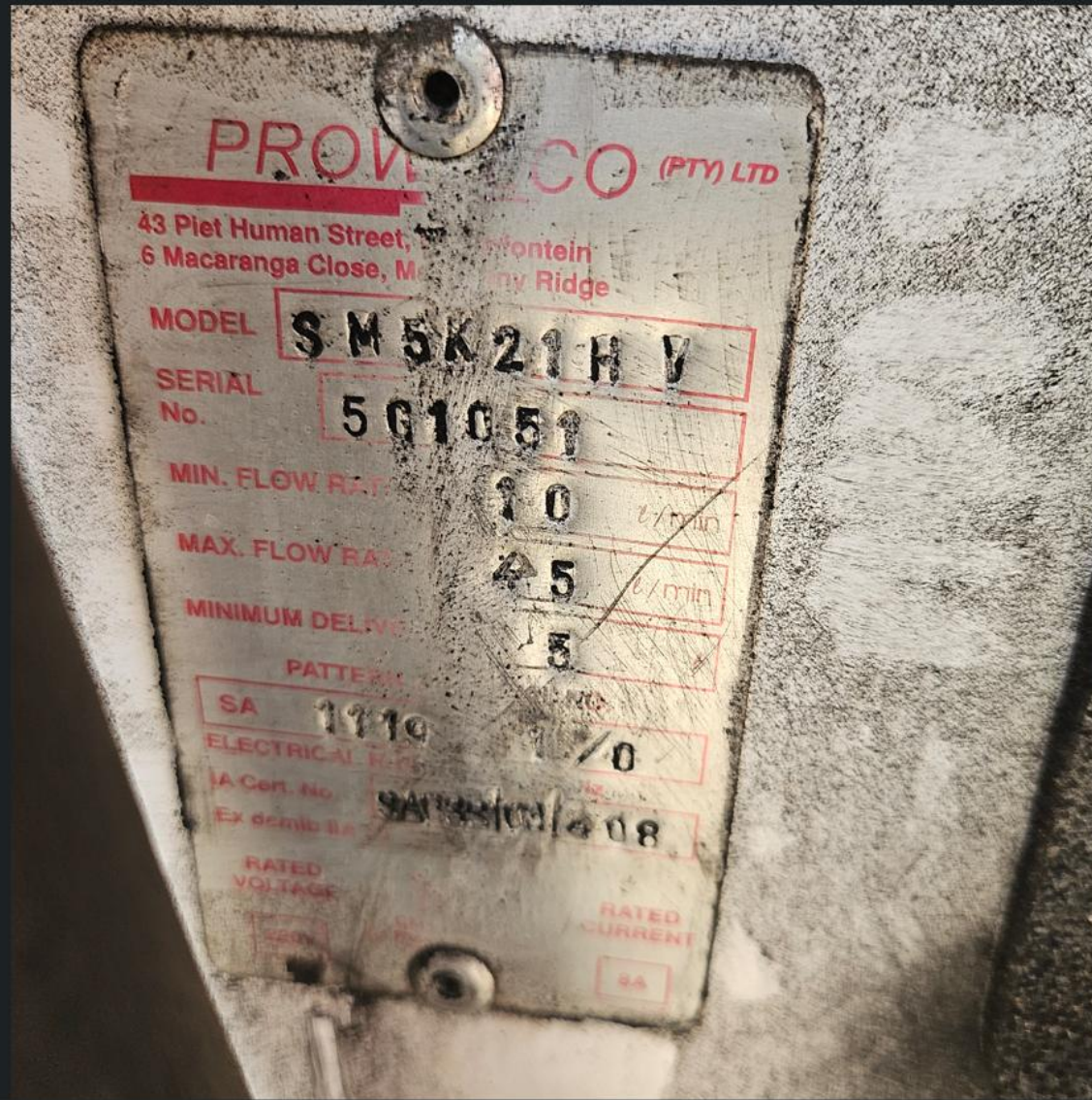
Dispenser Pump Nameplate.jpg
