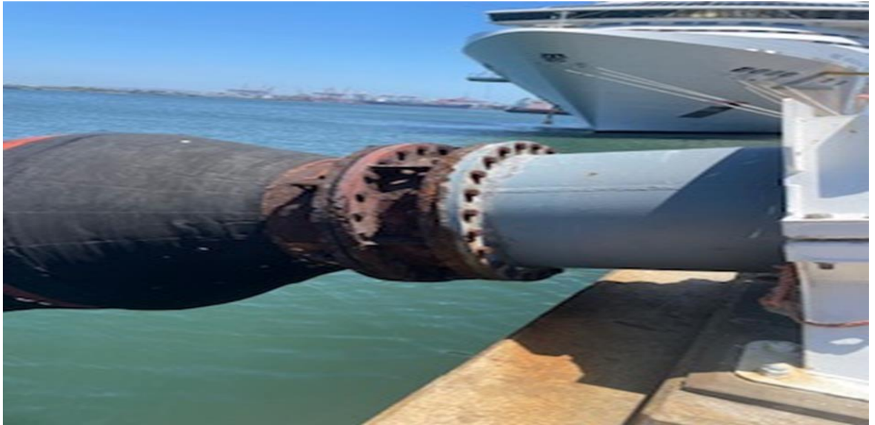
Rusted flanges: Require replacement of nuts and bolts plus denso tape.
