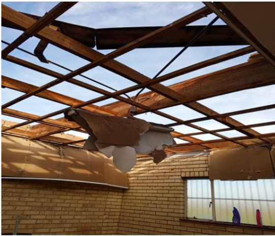
Figure 1: Damaged roof and ceiling
