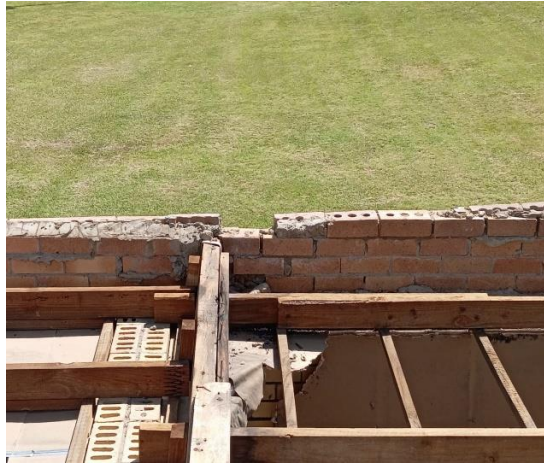
Figure 2: Damaged roof trusses and walls
