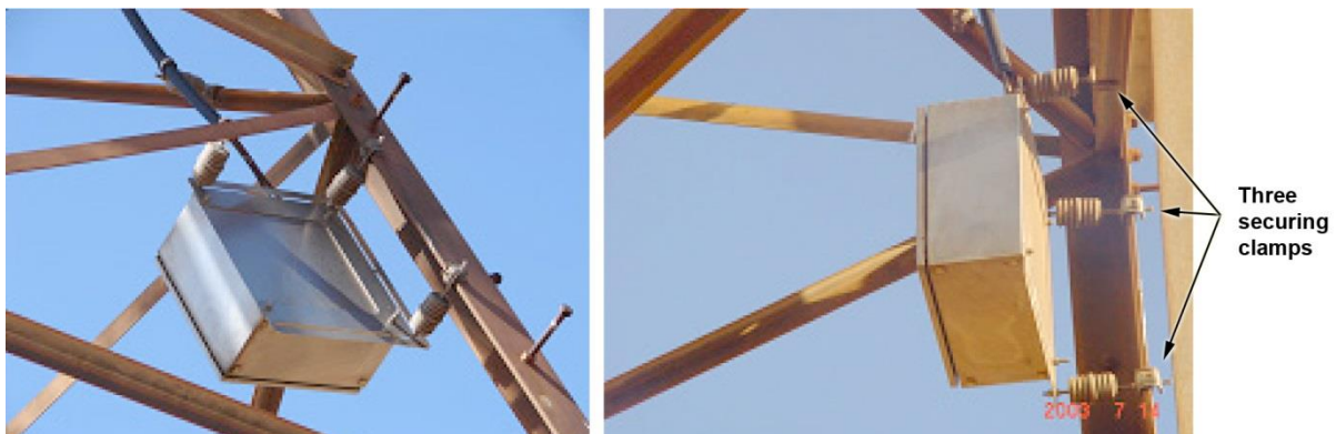
Figure 7: Joint Box Example (Insulated)
