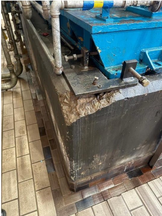
Figure 1: Spalled Concrete and Dislodged Anchor Bolt
