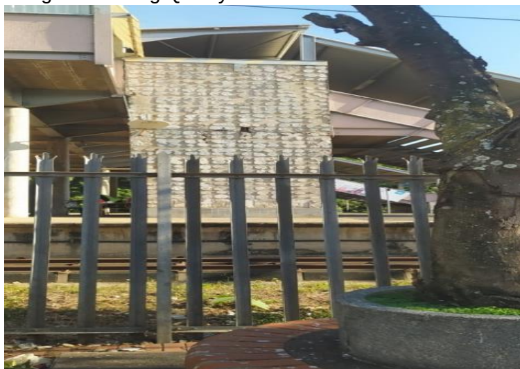
Image 6: Missing Quarry Tiles
