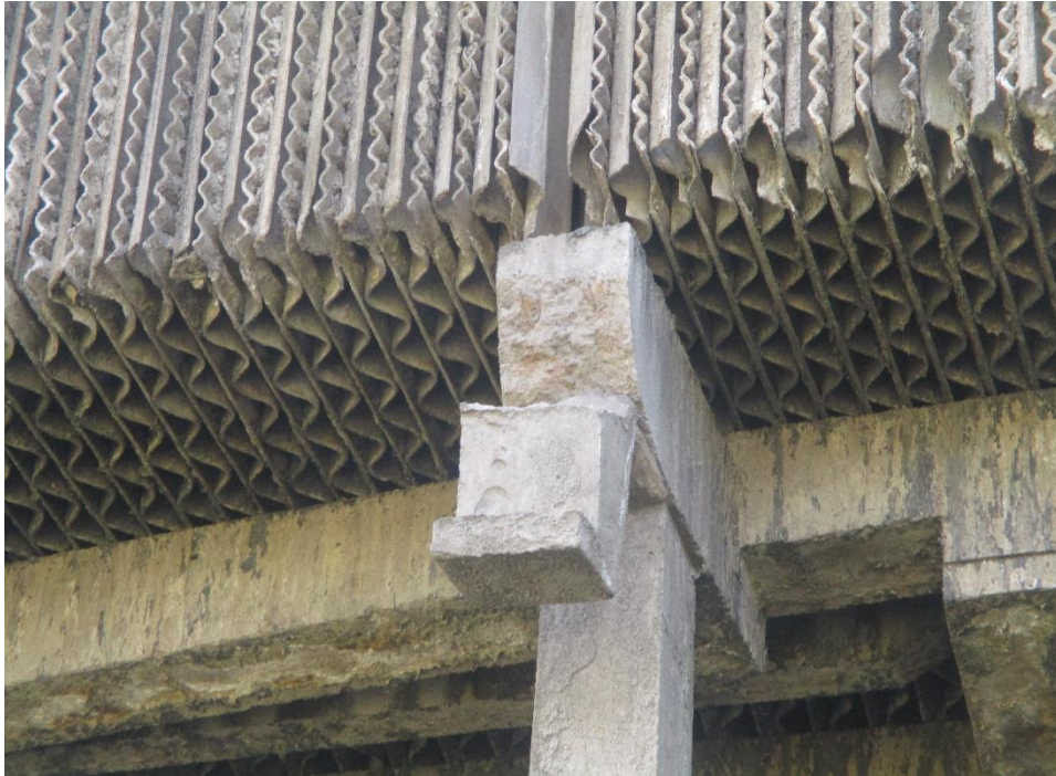
Photo 1: Failed precast concrete corbel
