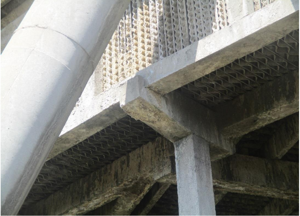
Photo 6: Cracked concrete corbel
