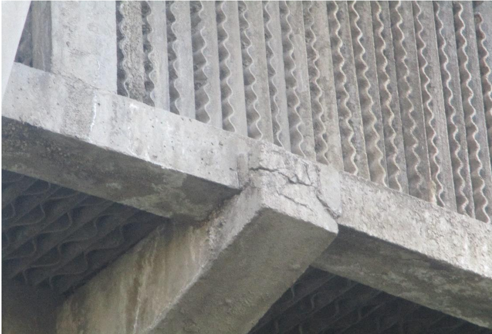
Photo 3: Concrete corbel spalling
