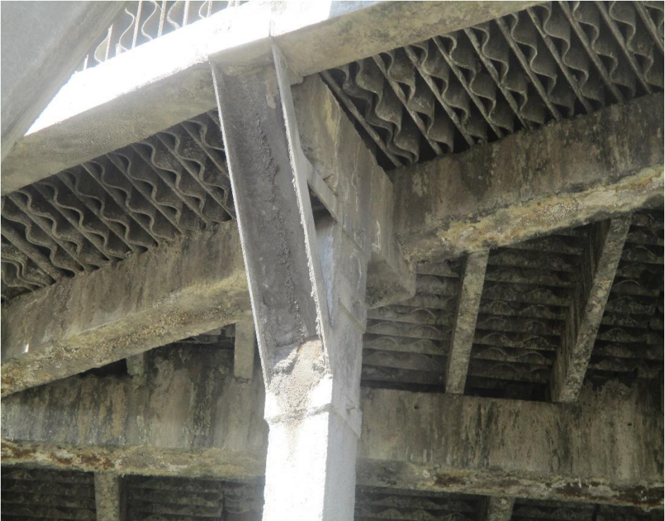
Photo 5: Rusted stainless steel knee-bracing - type B
