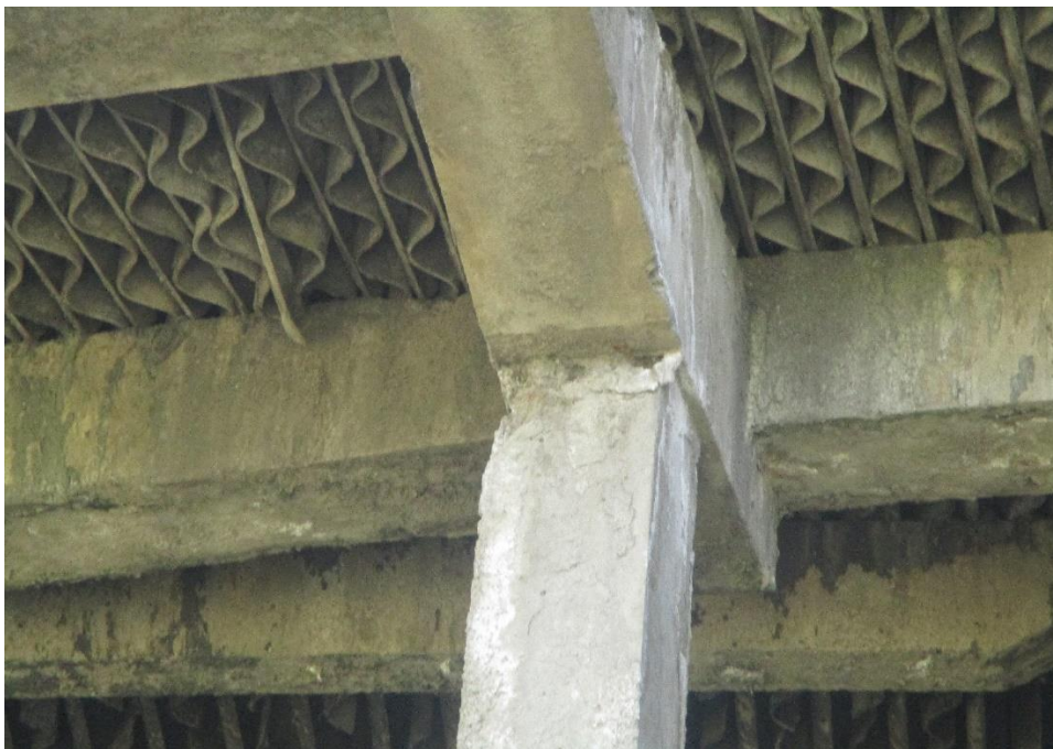
Photo 2: Evidence of concrete scaling between the beam and column
