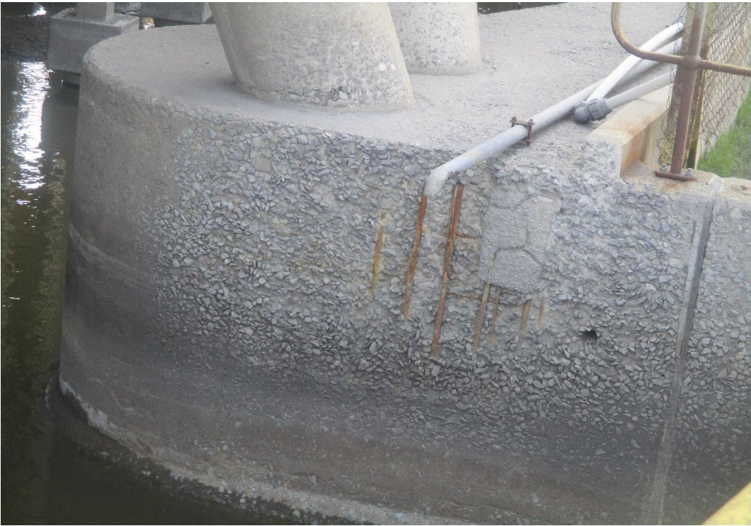
Photo 7: Scaling and corrosion on the concrete channel
