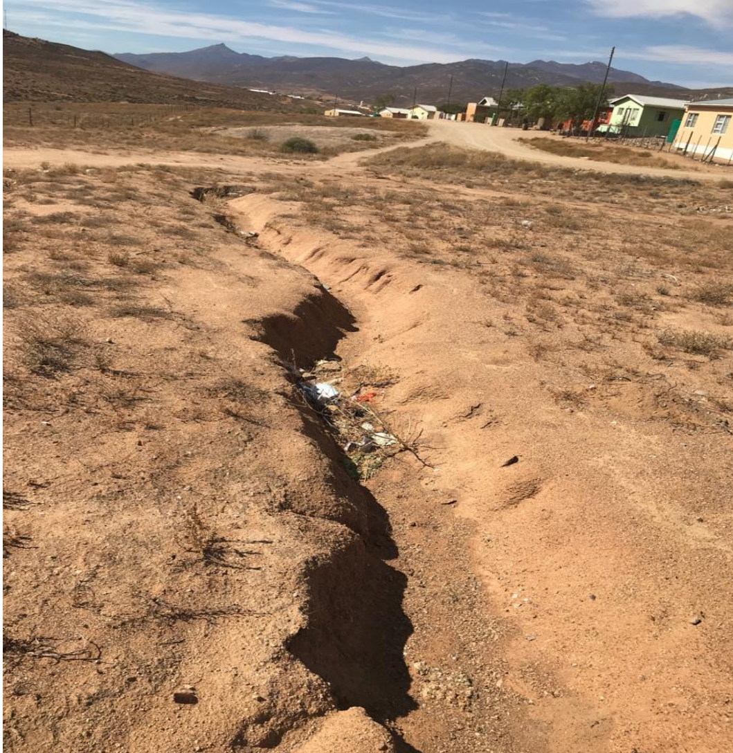
Figure 3: Showing the gulley erosion on site.
