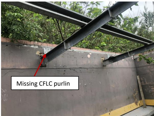
Photo 13: Missing CFLC purlin to be replaced.
