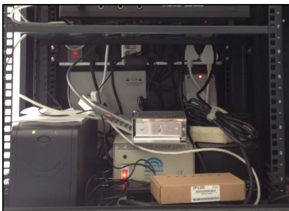
Figure 7: Example of Poorly Organised Security Equipment Cabinet
