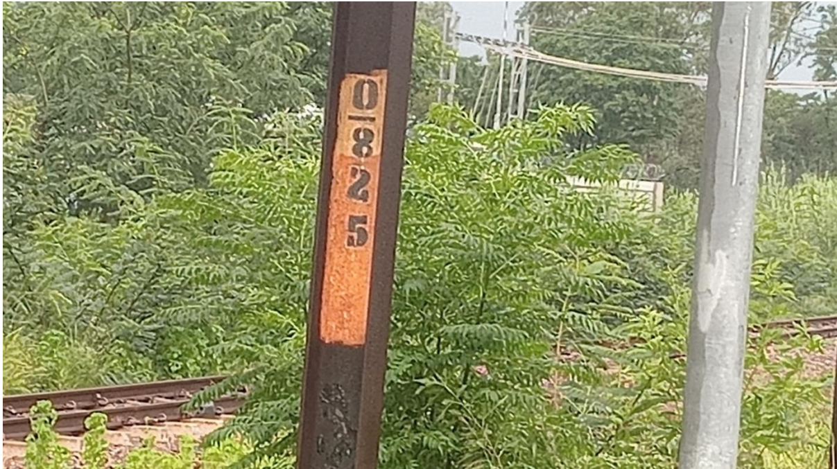
Figure 1: Mast pole number
