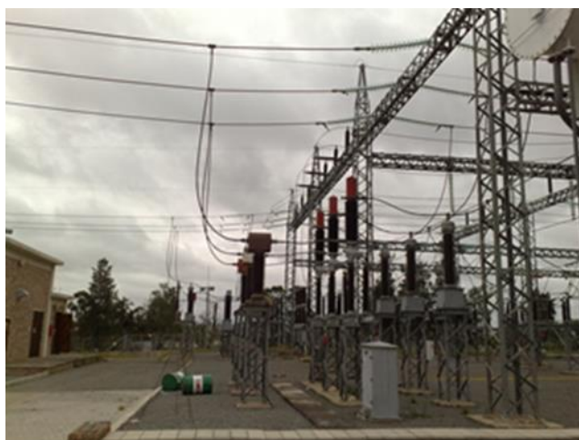
Kouga 2nd 66kV feeder bay at Melkhout Substation (ESKOM-EC Operating Unit)
