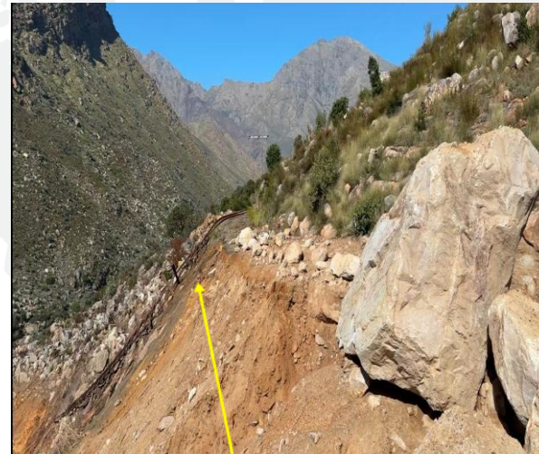
Washed Away Track Hanging down the embankment
