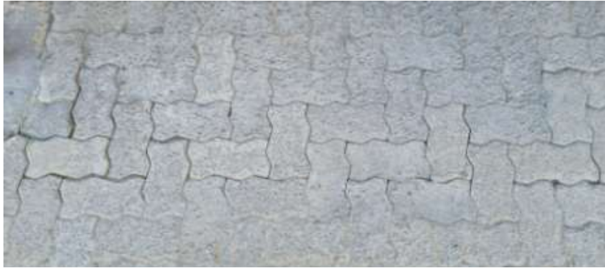
Figure 4: Lose of joint material
