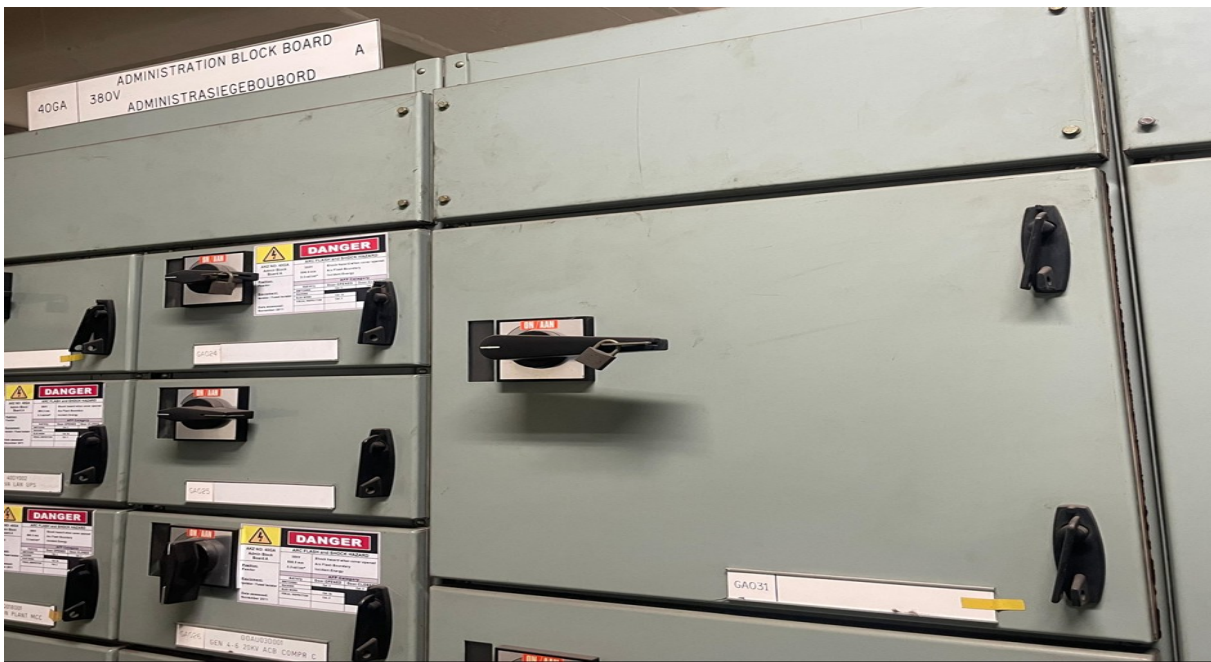
Figure 1: 380V Administration Block Board A (40GA)
