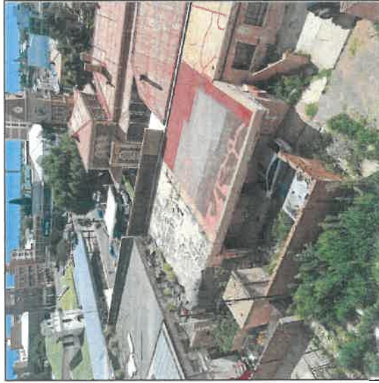
ROOF PHOTOGRAPH - HIGHLIGHTING DEFECTS NOT TO SCALE
