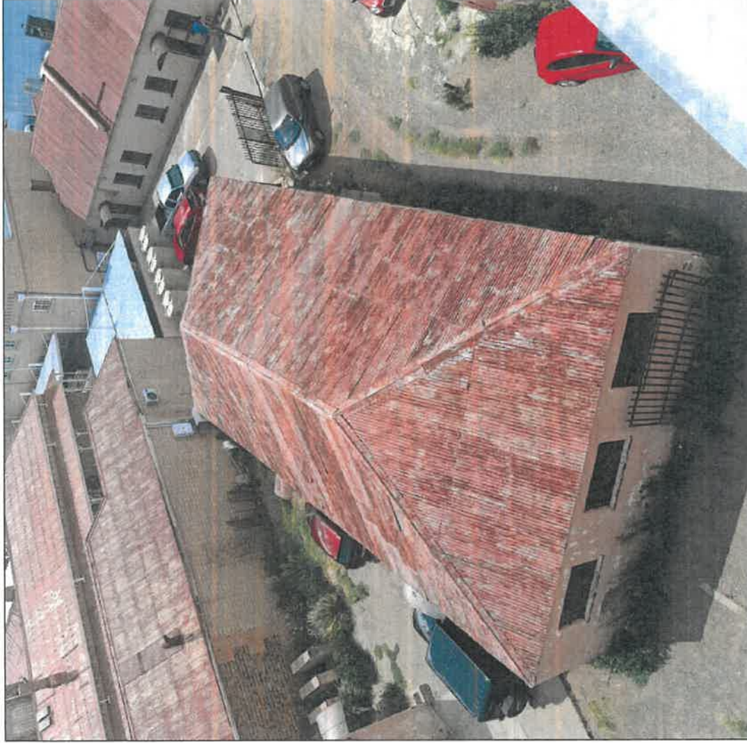
ROOF PHOTOGRAPH - HIGHLIGHTING DEFECTS NOT TO SCALE
