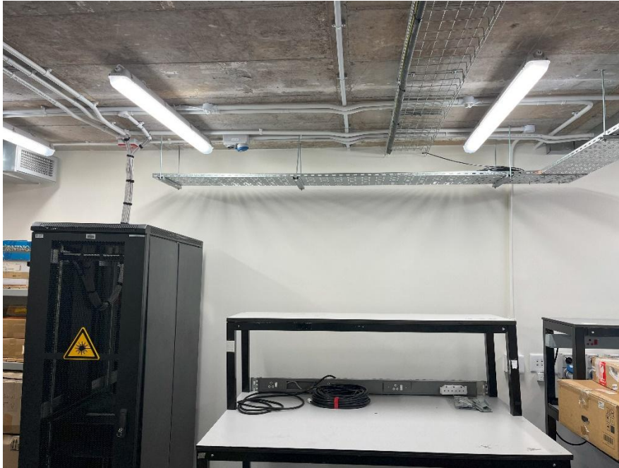
Figure 11: Tray near TFR laboratory Server Rack.
