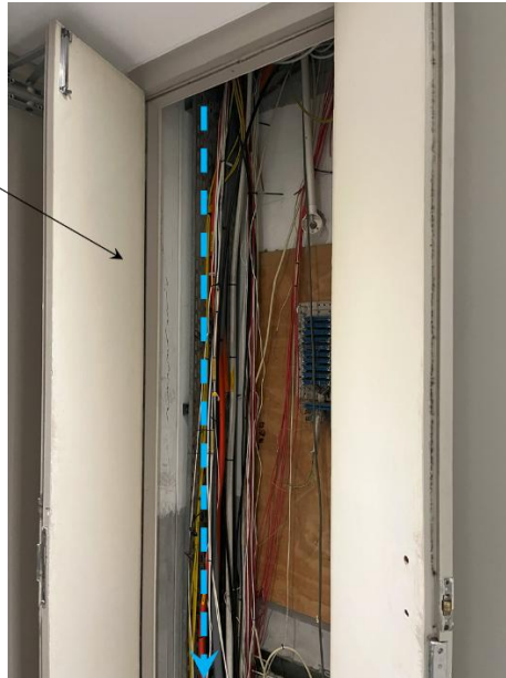
Figure 7: Cabinet located on the first floor of Liesbeek house.
