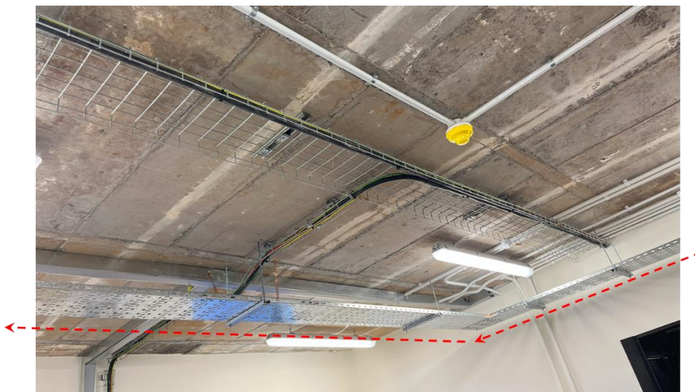
Figure 10: Cable tray located inside the TFR laboratory.
