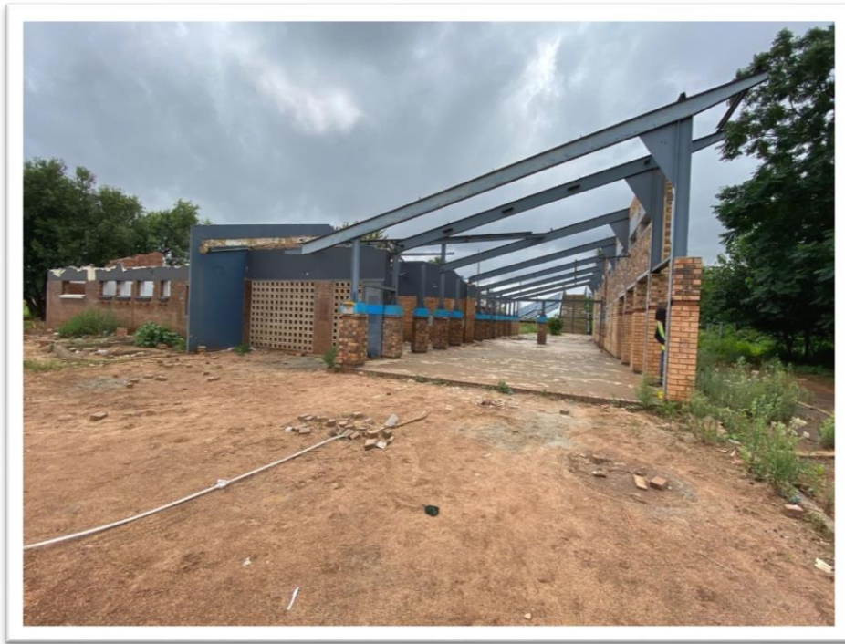
Building completely vandalized and its components stripped off.
