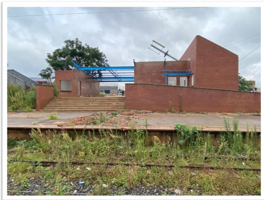
The building is completely vandalized, and its components stripped off.
