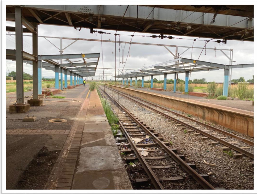
The roofs of all platform canopies are vandalized.
