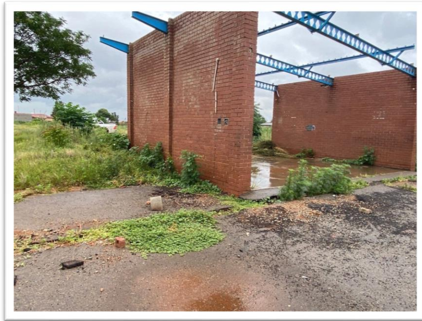
Entrance/Exit point completely vandalized.
