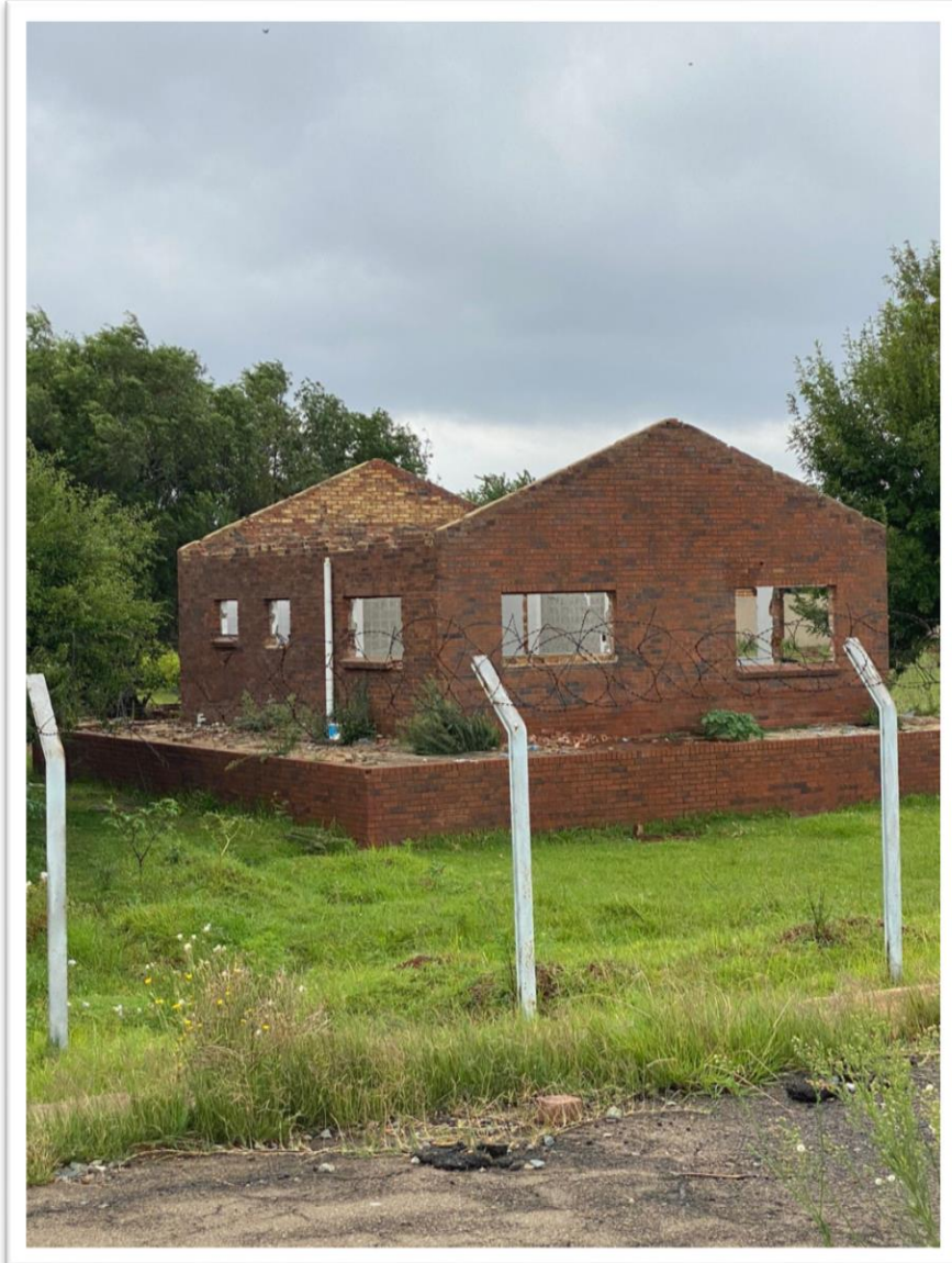
Building completely vandalized.
