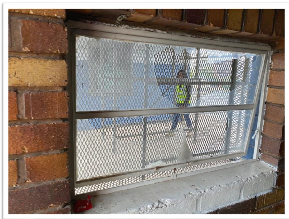
Broken window panes.
