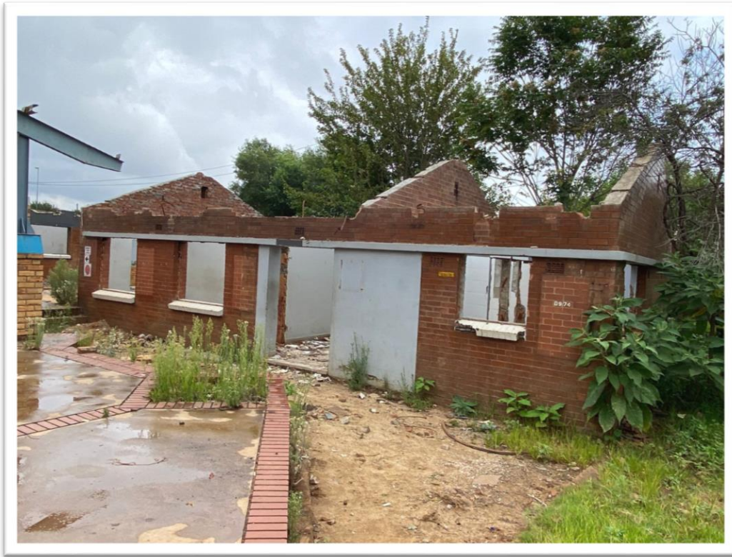
The building is completely vandalized.
