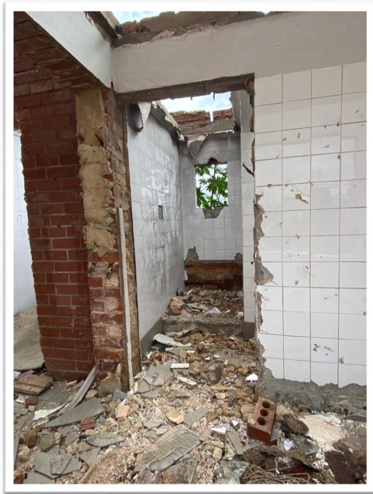
Inside the building is completely vandalized.
