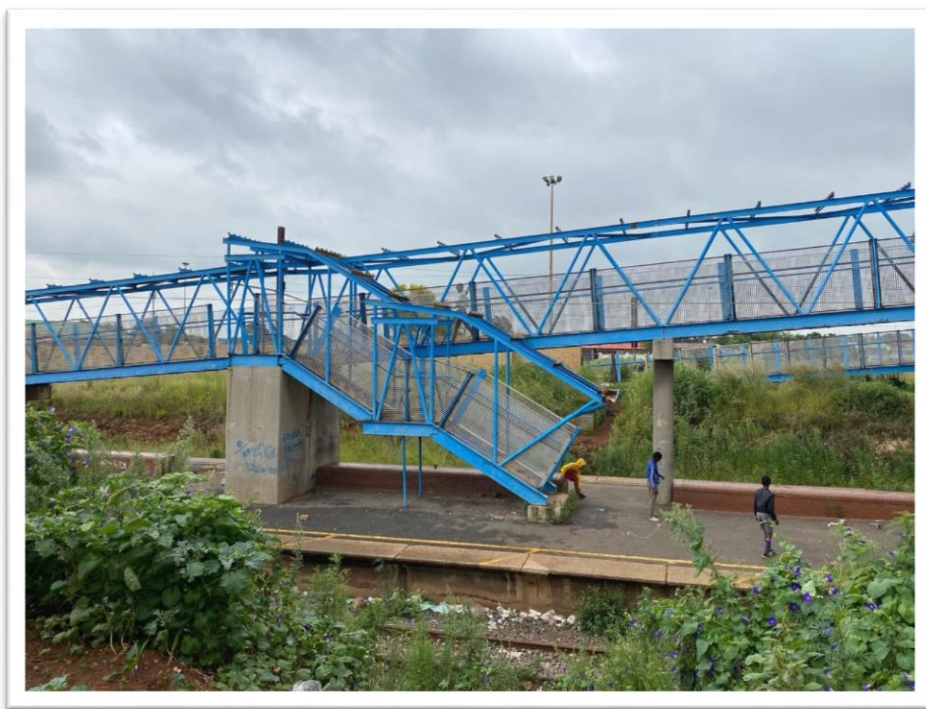
Suspended walkway vandalized.
