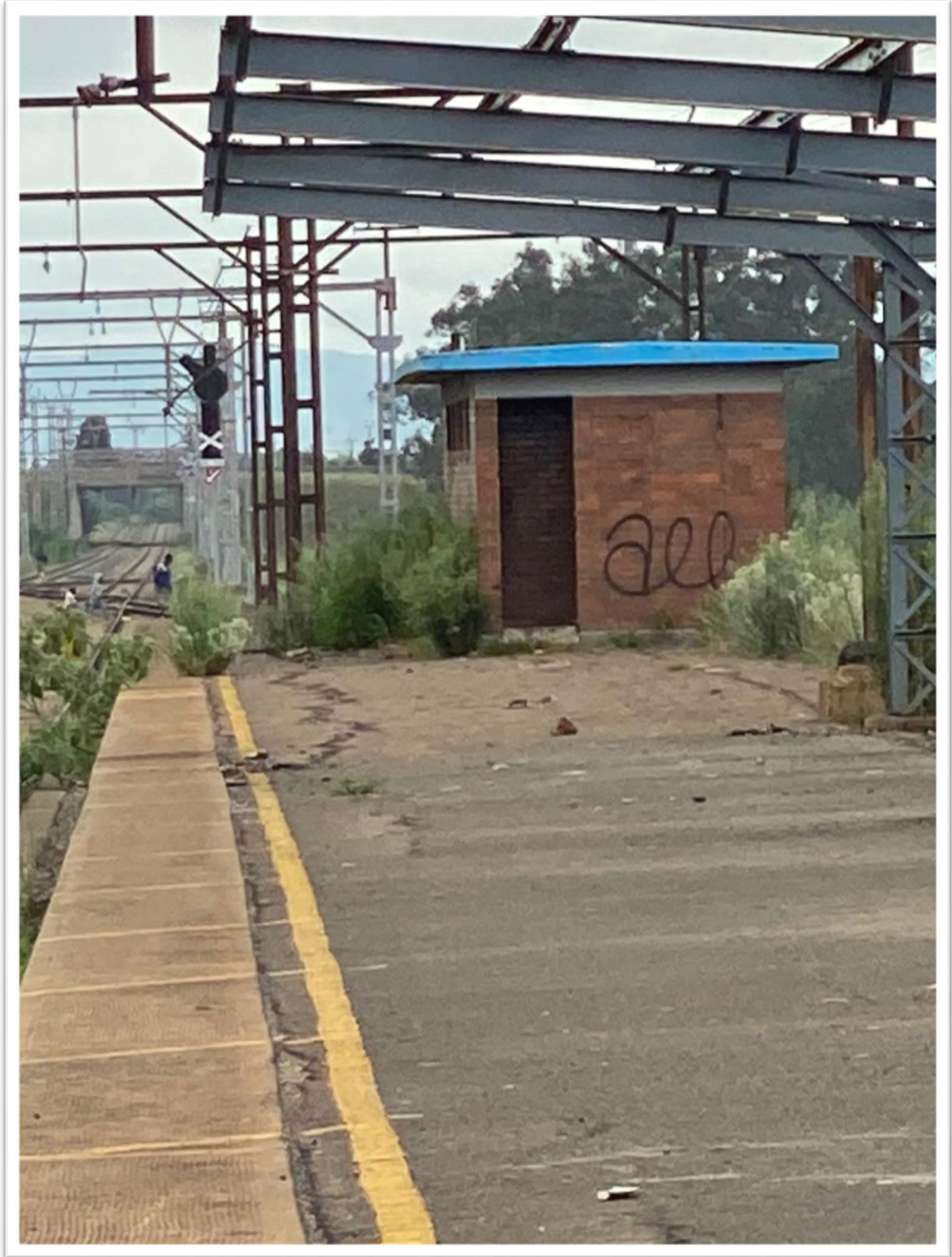
Building completely vandalized.
