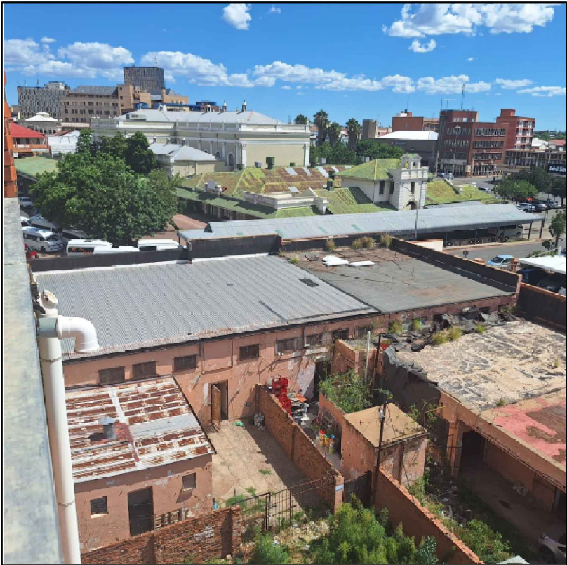
ROOF PHOTOGRAPH - HIGHLIGHTING DEFECTS NOT TO SCALE
