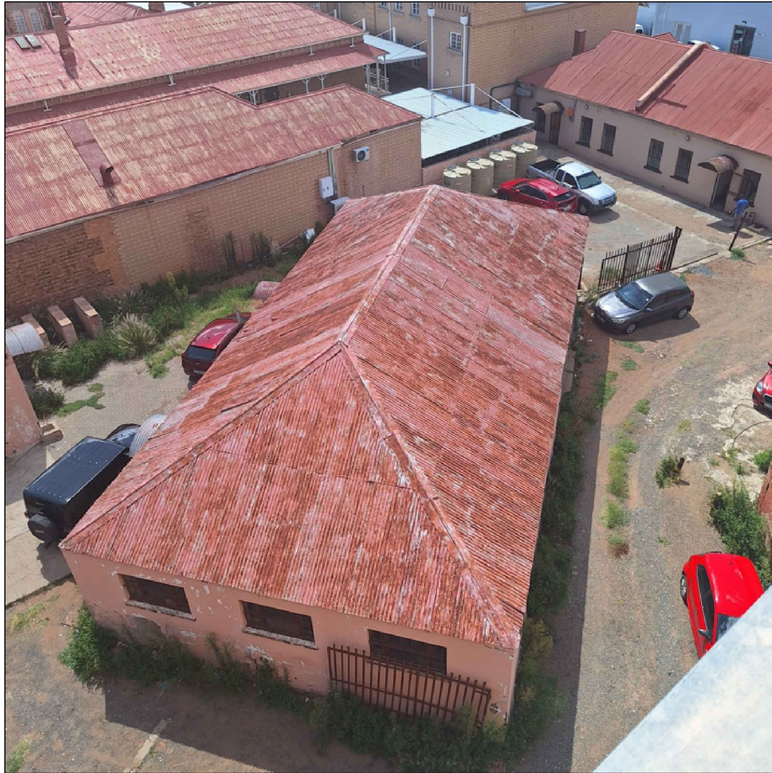
ROOF PHOTOGRAPH - HIGHLIGHTING DEFECTS NOT TO SCALE
