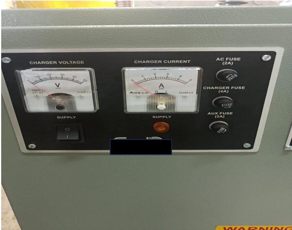
Picture 3. of 32 VDC, Amp meters, fuses and Volt meters.
