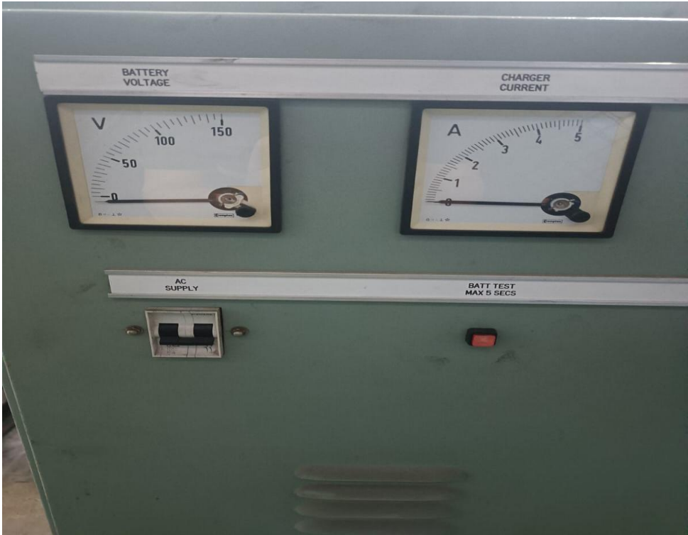
Picture 2. 110 VDC Amp meters and Volt meters
