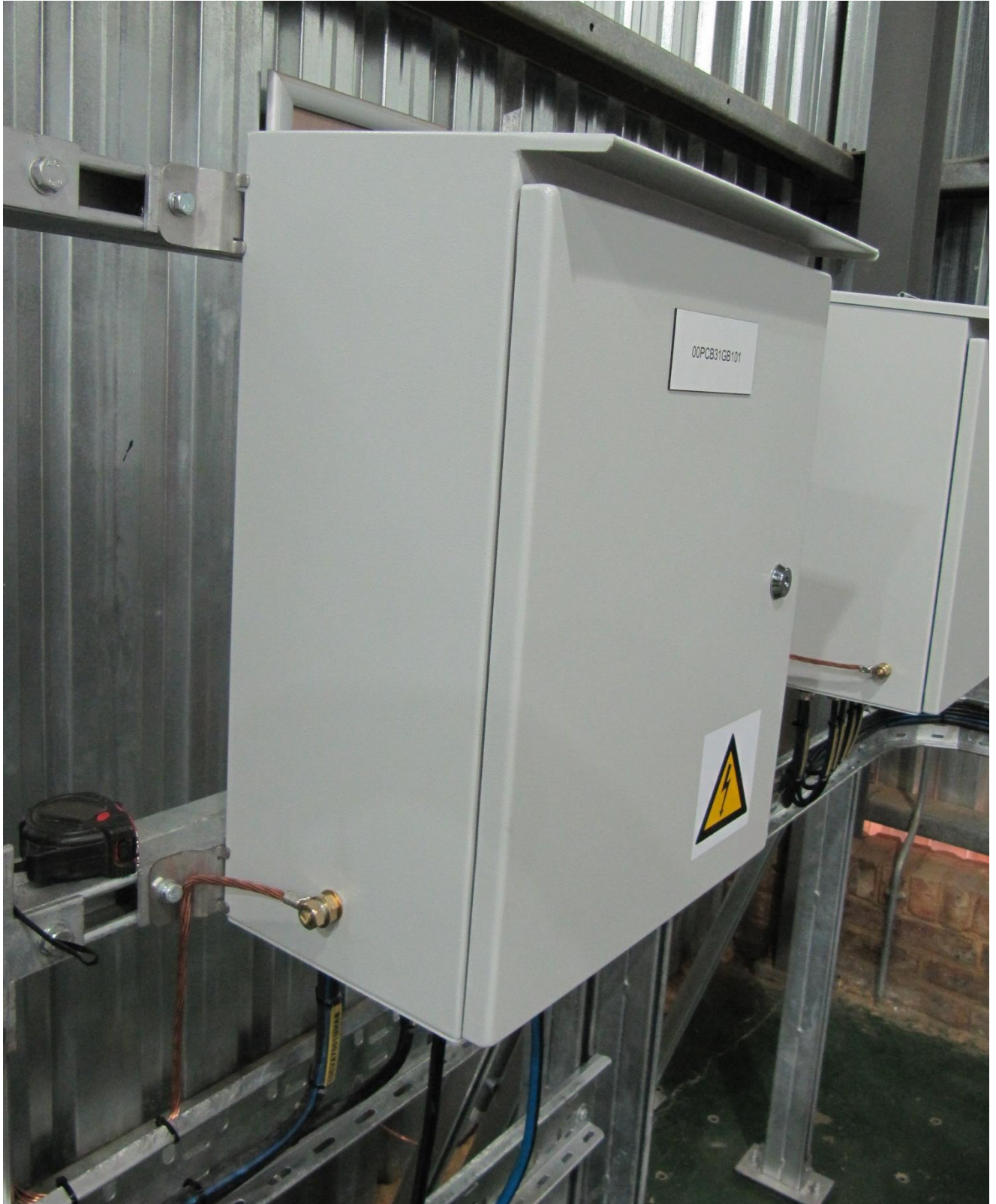
Figure 7: Typical Field Junction Box.
