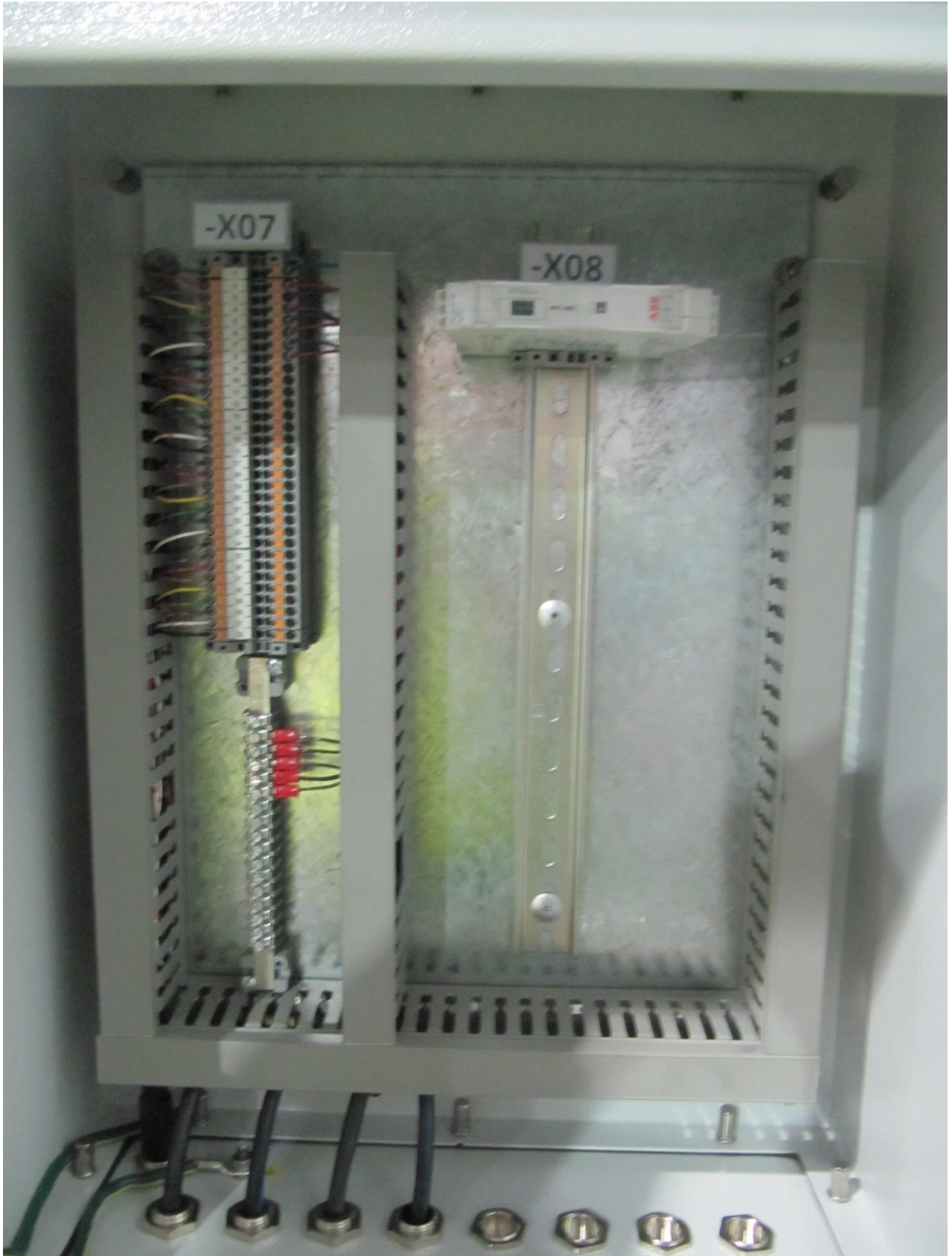
Figure 4: Inside of Typical Junction Box and Terminals.
