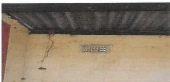
Figure 7: Picture of Internal Wall with crack
