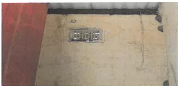
Figure 18: Picture of Internal Wall with crack
