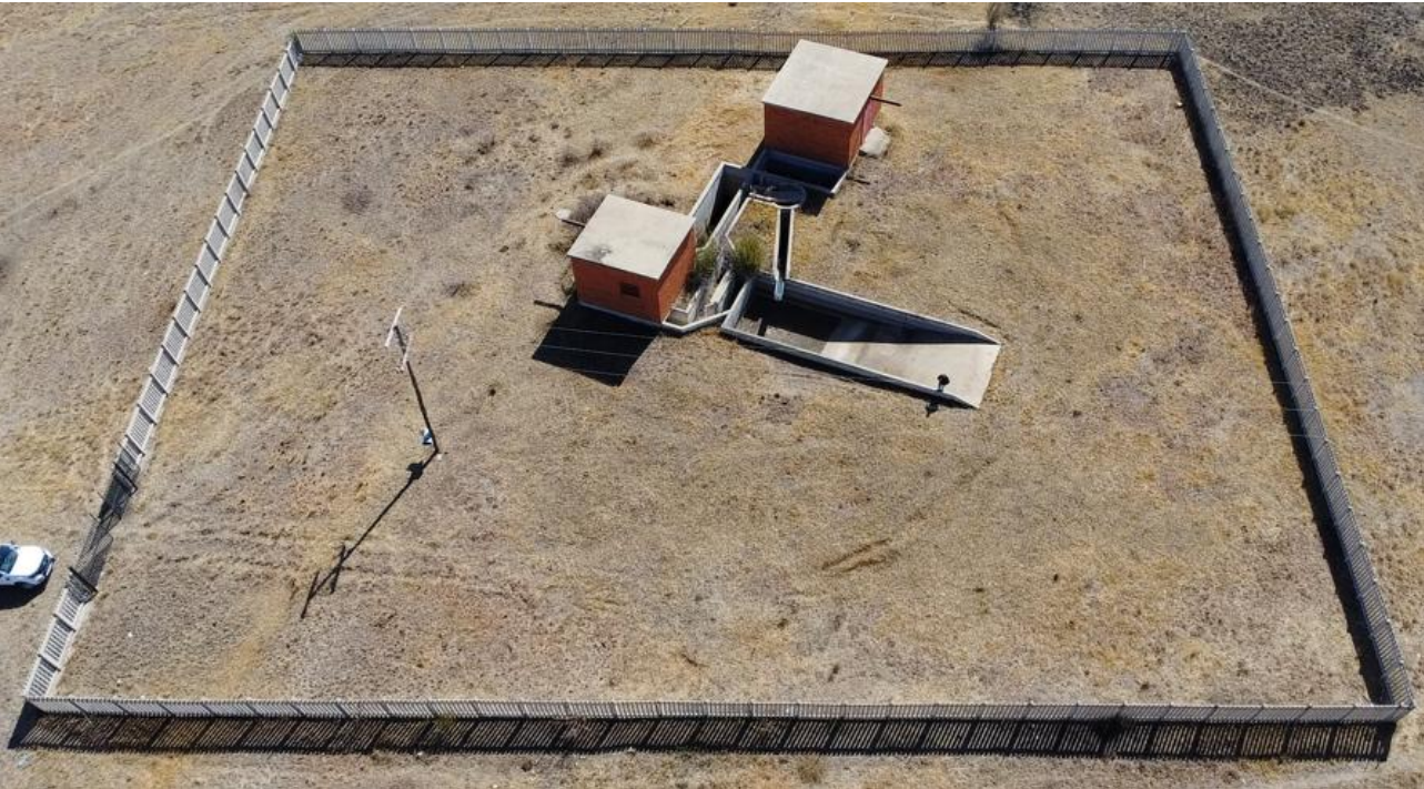
Existing Golf Course Pumpstation
