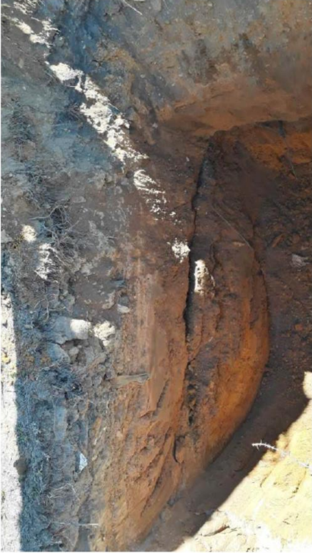
Photo 6 – View of subsoil profile as exposed in trial hole 3, note significant deposit of fill as well as slope instability due to saturation .
